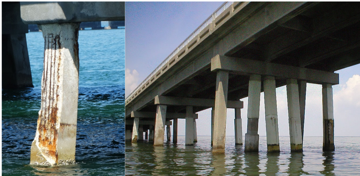
Figure 3. Corrosion damage near pile cap (left) and corrosion damage farther from high bending moment region (right).
