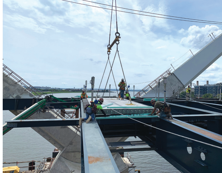
The Frederick Douglass Memorial Bridge used 480 precast concrete deck panels fabricated by Jersey Precast. Courtesy of South Capitol Bridge Builders.
