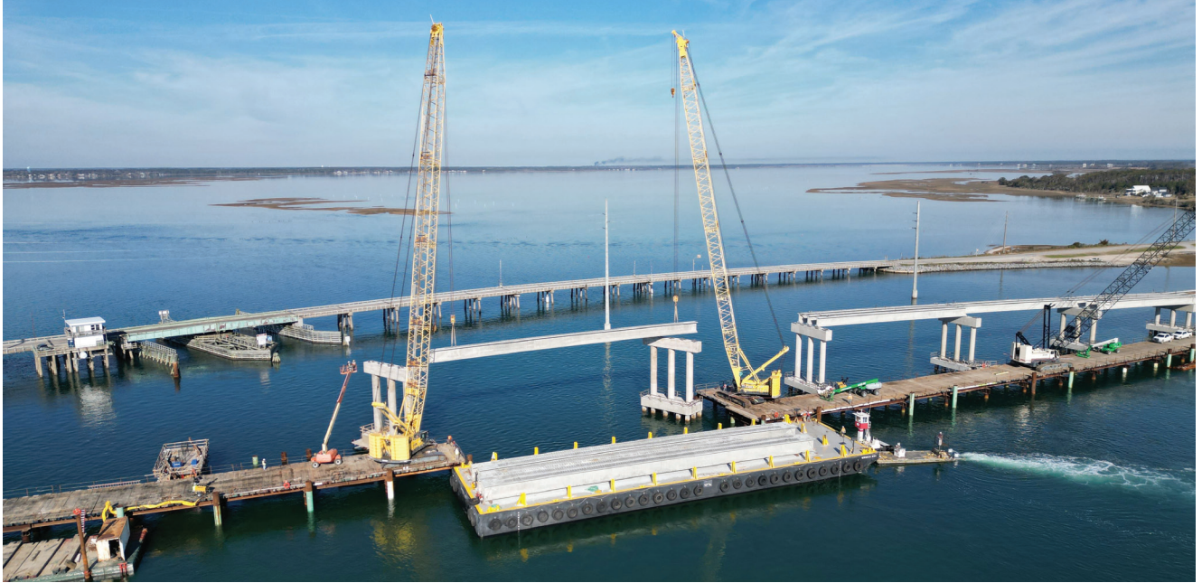
Many of the larger components for the new Earl C. Davis Memorial Bridge connecting Straits, N.C., with Harkers Island, N.C., were delivered by barge. Courtesy of Balfour Beatty Infrastructure Inc.
