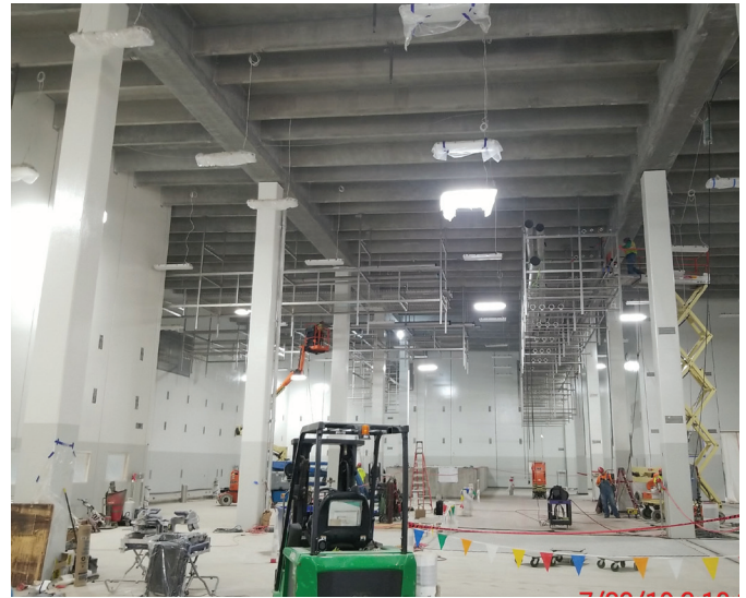
A 50 ft pipe rack is suspended from the structure and welded to embeds on the same day. Courtesy of Shambaugh & Son LP.
