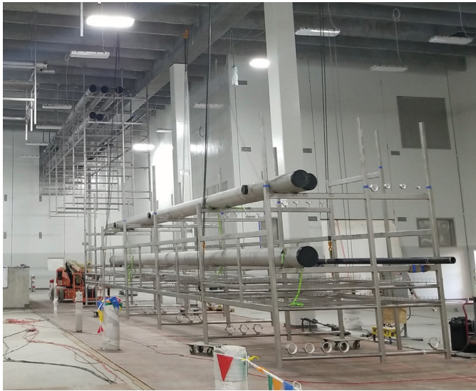
A 50 ft long pipe rack is staged for lifting in the morning. Note: 1 ft = 0.305 m. Courtesy of Shambaugh & Son LP.
