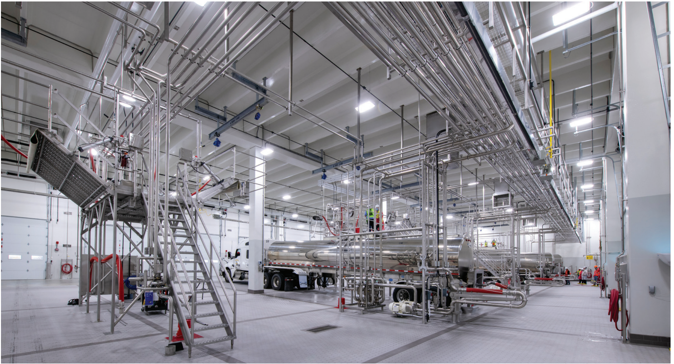
The final in-place construction is shown for the building and piping in the receiving area. Courtesy of Shambaugh & Son LP.
