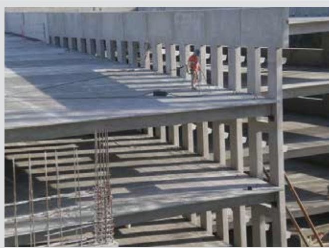
Figure 3. Precast concrete double-tee deck diaphragm. Image courtesy of Pat Hynes, Knife River Prestress Division, Harrisburg, Ore.
