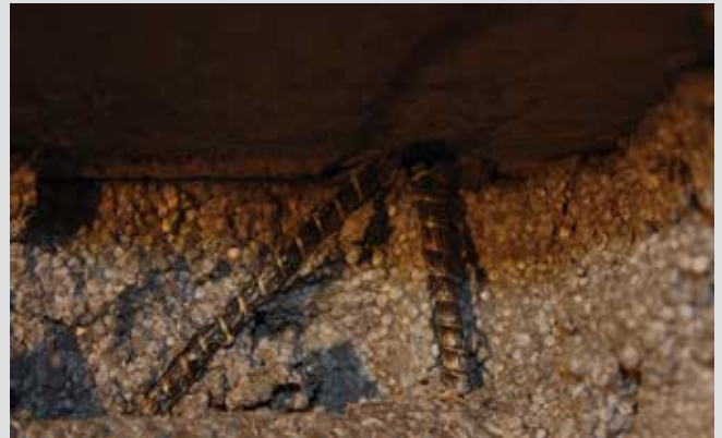
Failed shear connector in BPF
