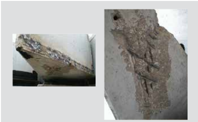
Figure 1. End damage observed on skewed bridge box beams during production.
