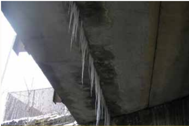
Figure 16. Leakage can occur through longitudinal joints. Photo courtesy of the Pennsylvania Department of Transportation.
