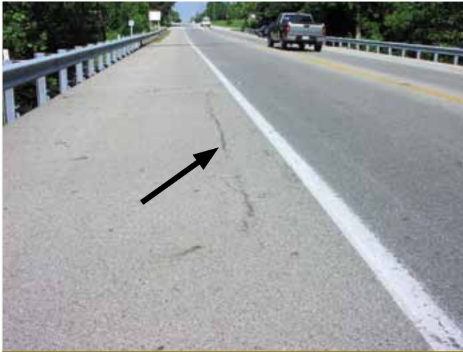
Figure 14. Longitudinal cracking can occur in an asphalt riding surface.
