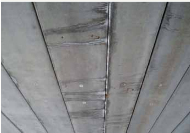
Figure 17. Efflorescence on the underside indicates leakage through the joints. Photo courtesy of the New York State Department of Transportation.
