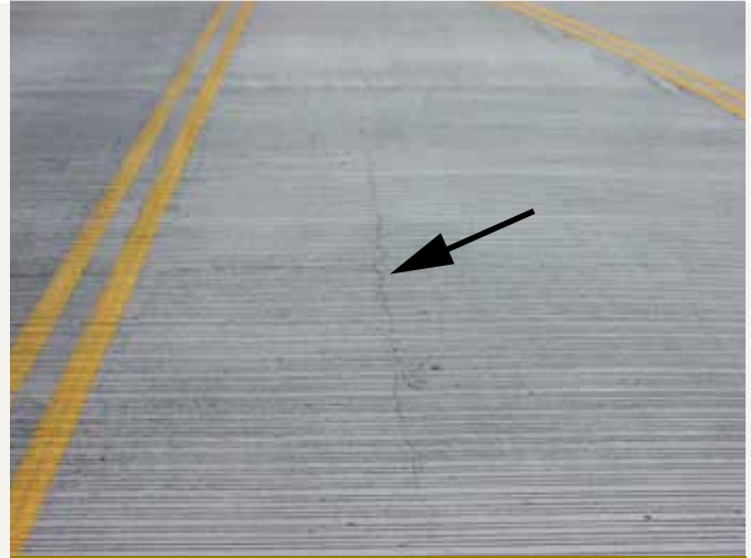
Figure 15. Longitudinal cracking can occur in a composite concrete deck.
