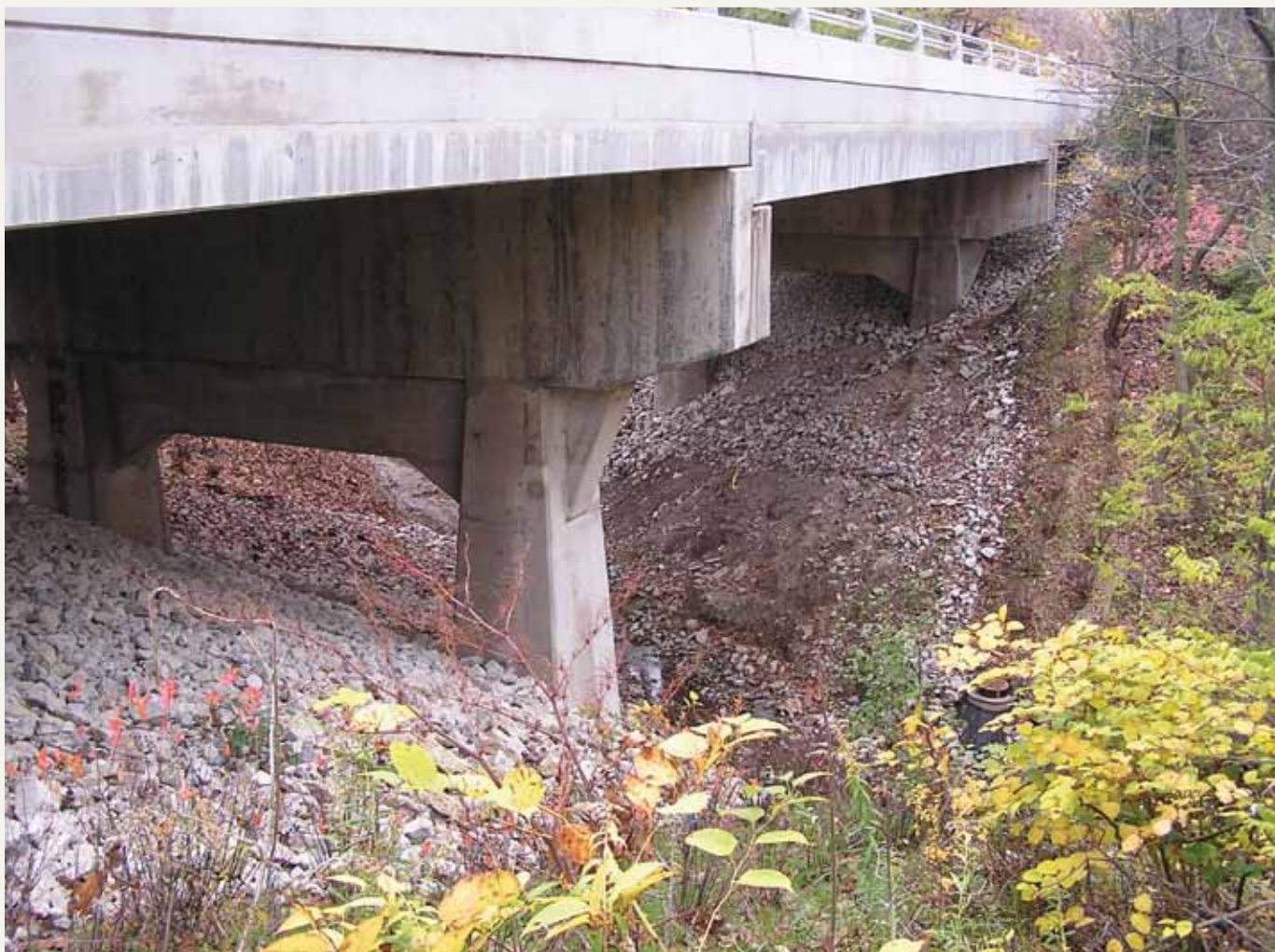
Figure 2. A three-span box-beam bridge was used over a ravine in Illinois. Photo courtesy of the Illinois Department of Transportation.
