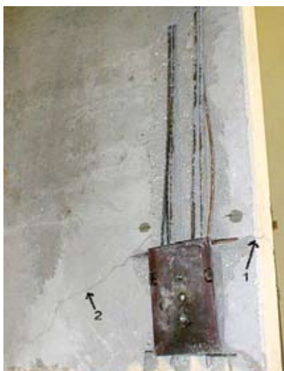
Fig. 23. Failure surface from base embed test.
