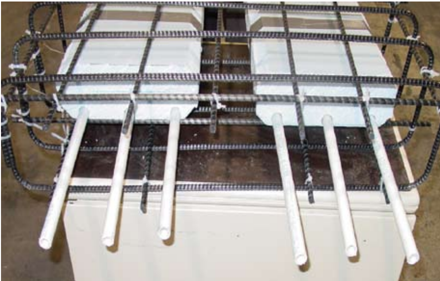
Fig. 2a. Close-up view of carbon fiber reinforced polymer reinforcement cage of box beam BBD-1.
