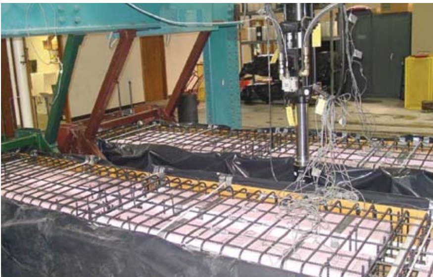
Fig. 2b. Carbon fiber reinforced polymer reinforcement cage for BBD-I placed in the formwork.
