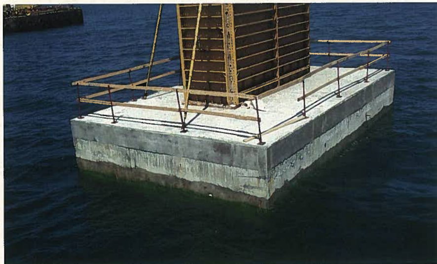
Fig. 6. View of a completed pile cap and hammerhead pier shaft with the temporary forms still in place.
