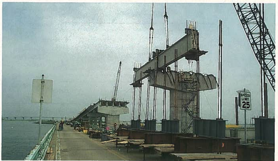
Fig. 11. Erection of precast concrete pier table girder with strongbacks already installed on the ends of the pier table girders.
