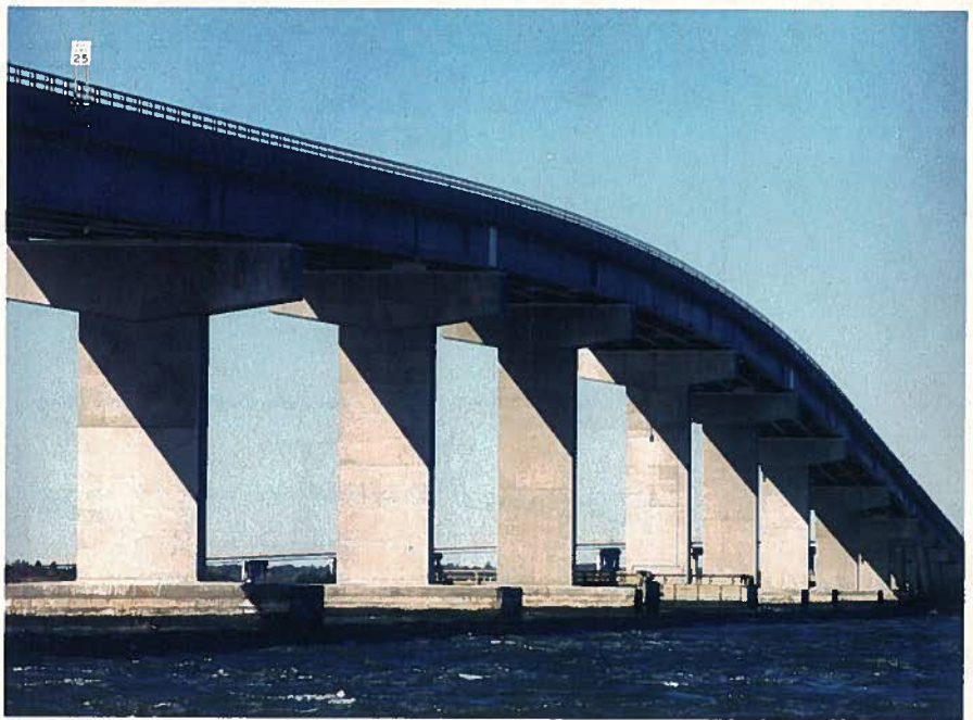
Fig. 8. Hammerhead piers founded on precast concrete cofferdam pile caps in rough waters. Photo courtesy: Gregg Kohl, AC Photo.
