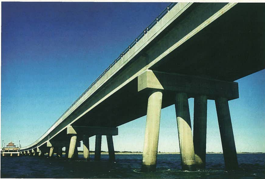
Fig. 5. Underneath view of the precast concrete piers for the shallow water foundations. A precast concrete system allowed for versatility and economy in the design of deep and shallow foundations. Photo courtesy: Gregg Kohl, AC Photo.
