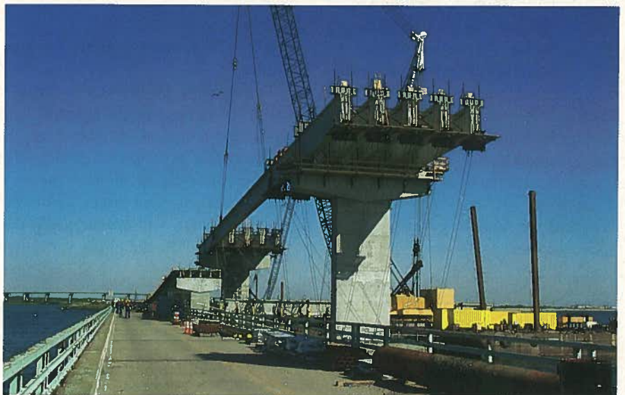
Fig. 12. Erection of precast concrete drop-in span girder; temporary blocking and bracing were left to the contractor.
