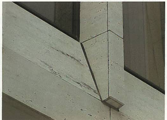
Fig. 21(b). Closeup of 1\frac{1}{4} in. (3 cm) travertine clad mullions meeting spandrel at third floor.
