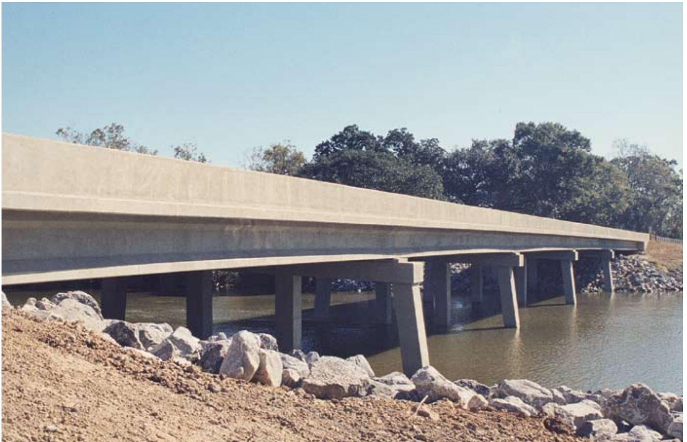
Fig. 7. The substructure consists of HPC bent caps supported by two sizes of piles using 10,000 psi (69 MPa) concrete.
