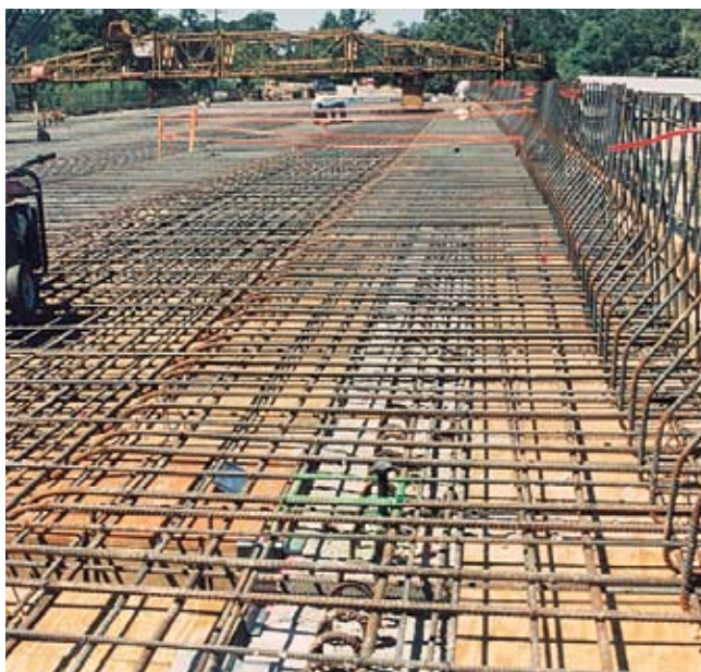
Fig. 12. Sections of reinforcing bar were marked (with red flagging and green print) to indicate where the instrumentation would be placed.
