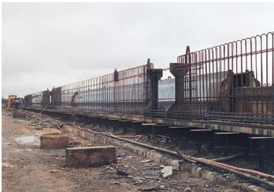
Fig. 8. The five precast, prestressed girders for each span were cast in a line at the same time.
