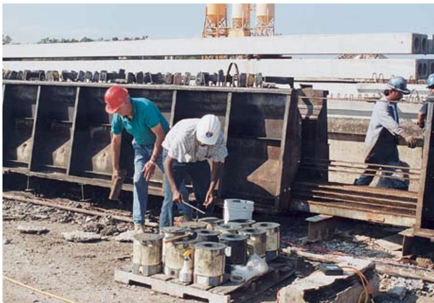
Fig. 9. Cylinder testing was done continuously to ensure compressive strengths were being met. In background, newly cast prestressed concrete piles can be seen.
