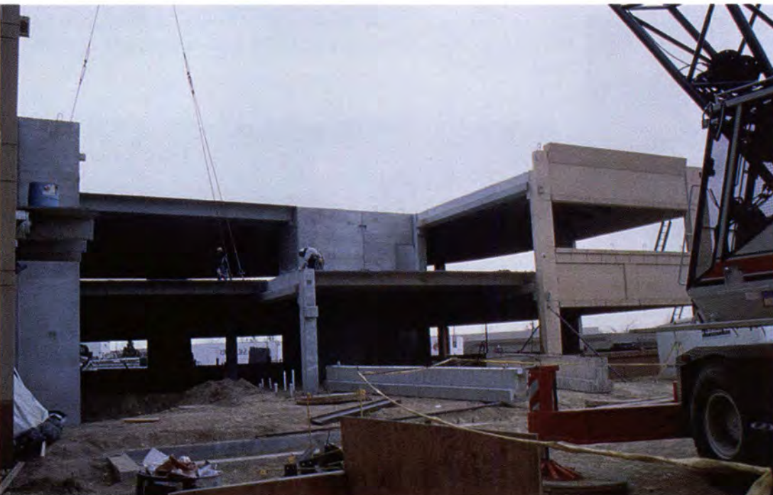
Fig. 40b. Construction showing use of columns and spandrels in Interlocken Office Campus.
