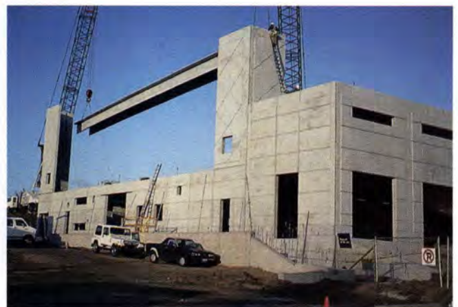
Fig. 49b. Erection of main roof system consisting of 40½ in. (1029 mm) deep lightweight double tees spanning 111 to 140 ft (34 to 43 m) from bearing wall to bearing wall (United States Olympic Training Center, Colorado Springs, Colorado).
