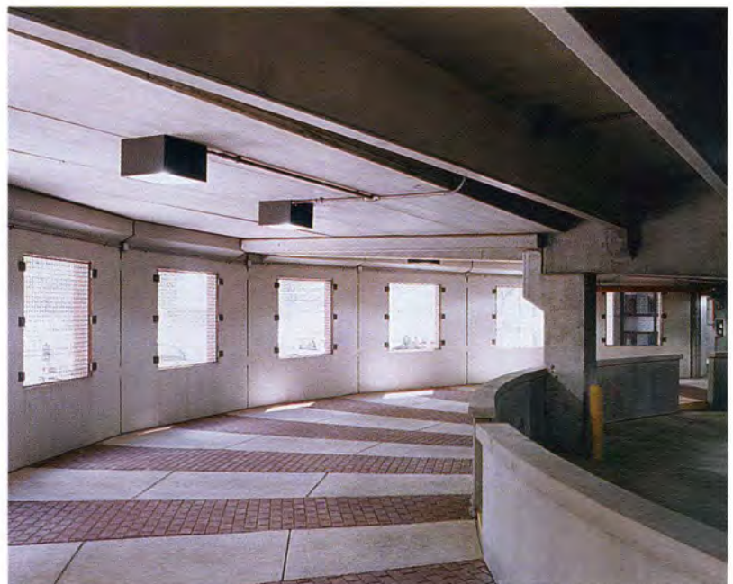
Fig. 46b. Hollow-core units supported by walls in walkway areas (Jefferson Avenue Parking Structure, Detroit, Michigan).
