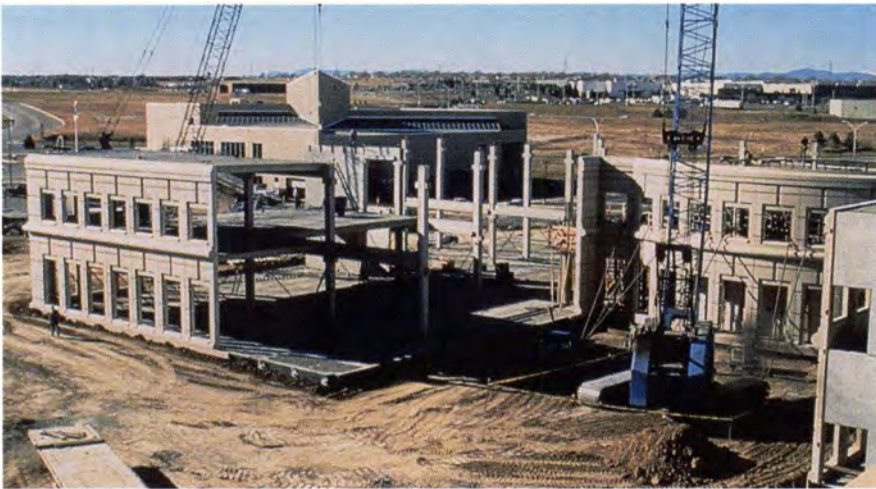
Fig. 45a. Two-story window wall units supporting double tees for Aurora, Colorado Municipal Justice Center, Aurora, Colorado.
