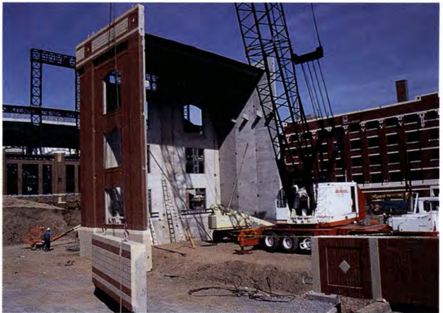
Fig. 4. The brick-faced precast panels on the Barker Substation, Denver, Colorado are 36 ft (11 m) tall.
