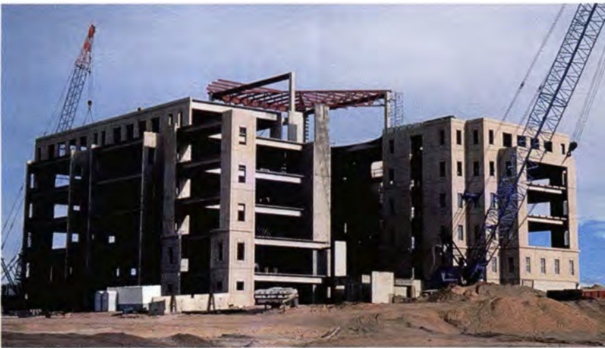
Fig. 43b. Construction showing window box panels supporting double-tee floor and roof members (Shepard's/McGraw-Hill World Headquarters, Colorado Springs, Colorado).
