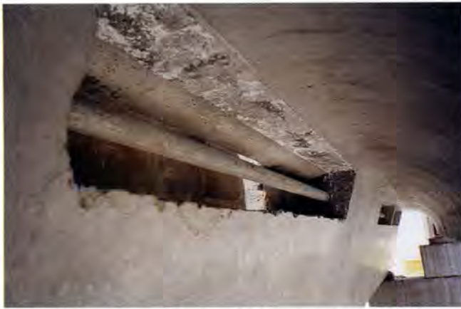
Fig. 8. Underside of triple riser (Viñoly stadia) shows steel braces that were added through center of opening to provide stiffness. Openings provided extra lighting for the concourse below.
