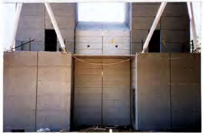
Fig. 16. Side of perimeter building with steel posts supporting the upper precast concrete risers already connected.
