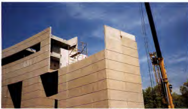
Fig. 15. A crane was used to erect the precast panels comprising the perimeter building surrounding the seating elements. The perimeter structure consists of both loadbearing and non-loadbearing panels, and hollow-core slabs.
