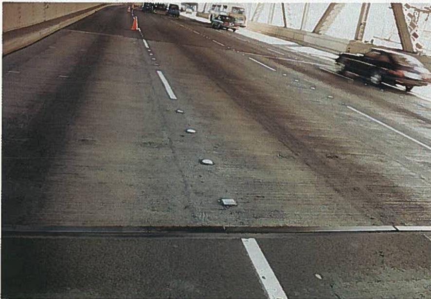
Fig. 11. Section of deck replaced due to earthquake, Oakland-San Francisco Bay Bridge, California.
