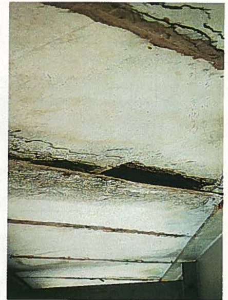
Fig. 19. Random cracking and spalling in Harriman Interchange Bridge, Orange County, New York.
