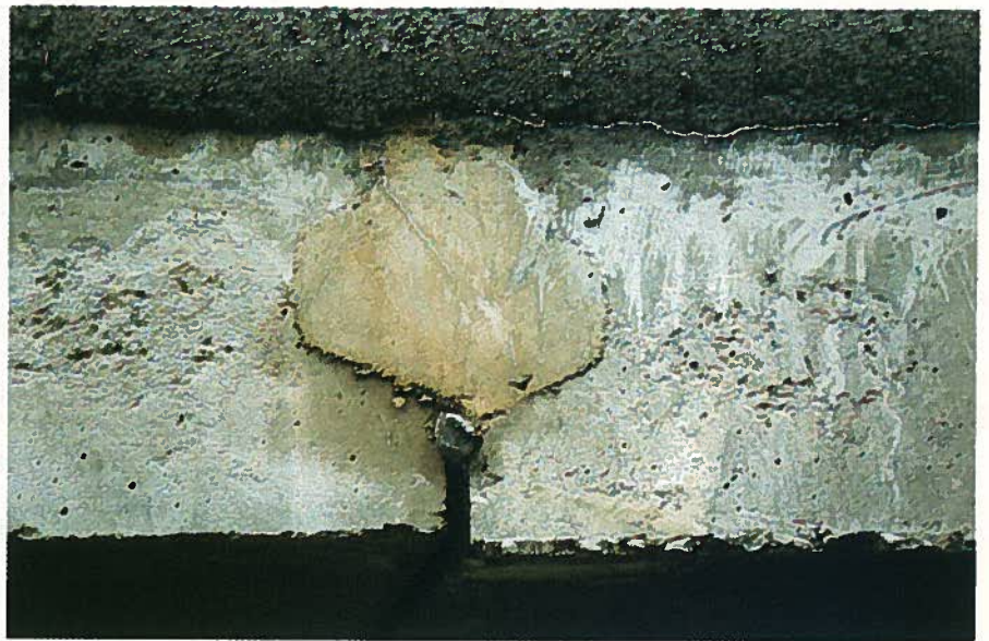
Fig. 32. Minor debonding at transverse joints, Chulitna River Bridge, Alaska.
