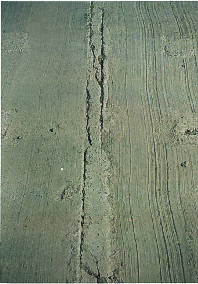
Fig. 36. Cracking and loss of material at transverse joints, Dalton Highway Bridges, Alaska.
