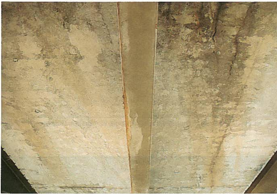
Fig. 6. Cracking and leaching in William Preston Jr. Memorial Bridge, Chesapeake Bay, Maryland.
