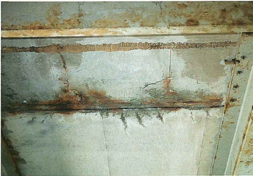
Fig. 17. Leaking and rusting in Amsterdam Interchange Bridge, Montgomery County, New York.
