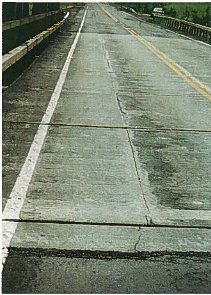
Fig. 25. Cracking in asphalt surface on Route 155 Bridge, Albany County, New York.
