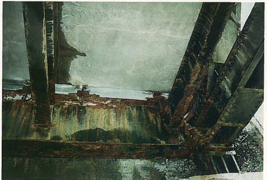
Fig. 24. Leaking at the transverse joints in Route 155 Bridge, Albany County, New York.
