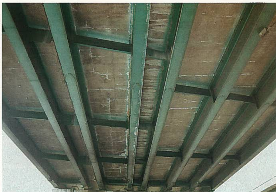
Fig. 9. Condition of deck and supporting system viewed from below, High Street Overhead Separation Bridge, California.
