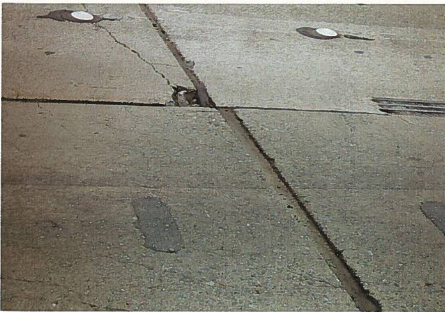
Fig. 10. Condition of deck and joints in High Street Overhead Separation Bridge, California.
