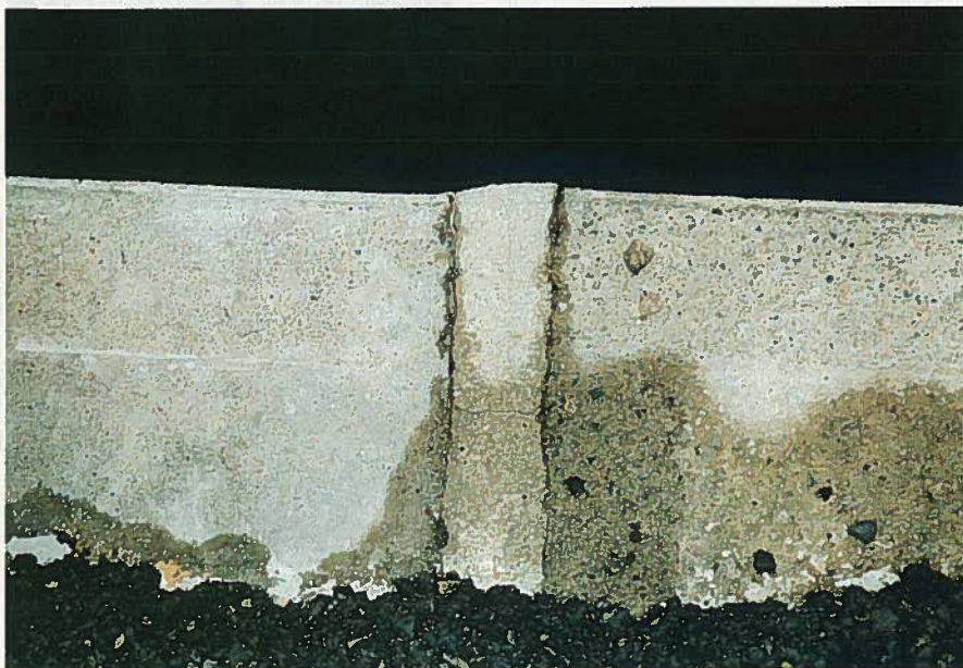
Fig. 22. Debonding in transverse joint in Batchellerville Bridge, Saratoga County, New York.
