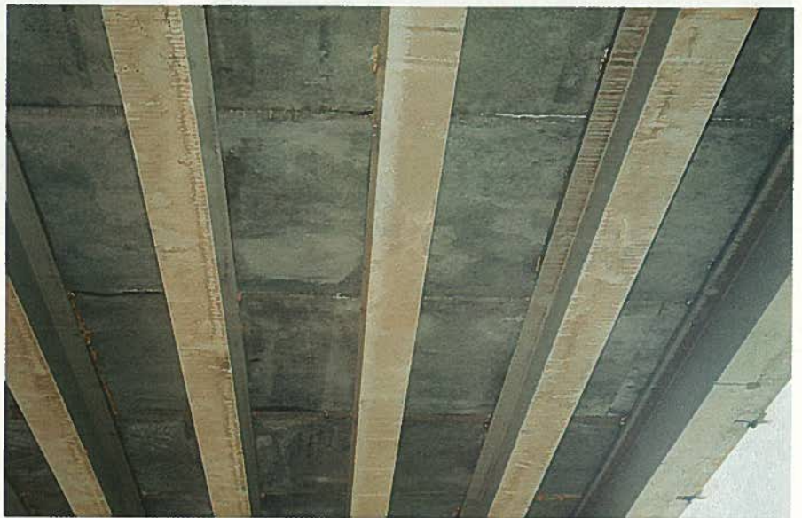
Fig. 35. Typical underside view of deck condition, Dalton Highway Bridges, Alaska.
