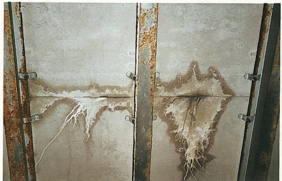
Fig. 44. Excessive leakage at transverse joints, B-501 Bridge, Somerset County, Pennsylvania.
