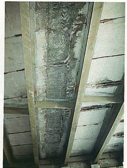
Fig. 13. Fracture and spalling at transverse joint in Krumkill Road Bridge, Albany County, New York.
