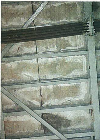
Fig. 27. Leaking underneath bridge deck, Kingston Bridge, Ulster County, New York.
