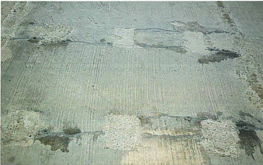
Fig. 38. Patching at shear connecting pockets, Dalton Highway Bridges, Alaska.
