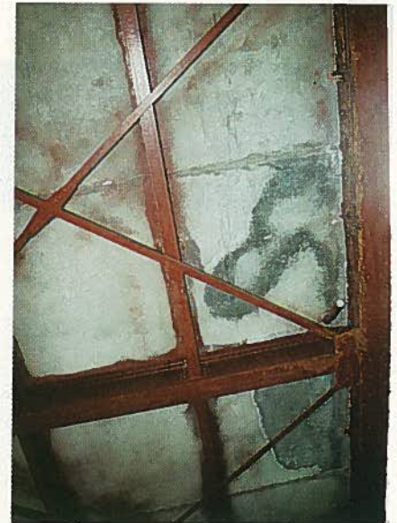
Fig. 20. Minor leaking in Vischer Ferry Road Bridge, Schenectady County, New York.
