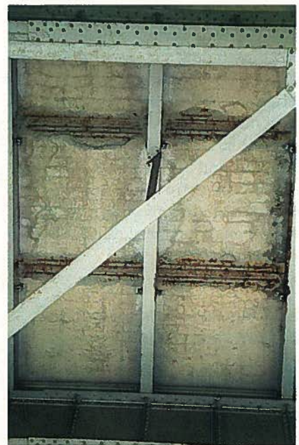
Fig. 48. Cracking and spalling, NB-750 Clark Summit Bridge, Lackawanna County, Pennsylvania.
