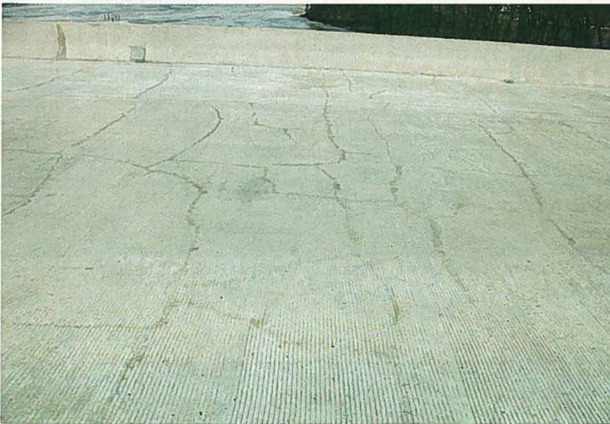
Fig. 7. Condition of overlay on Burlington Bridge, Iowa.
