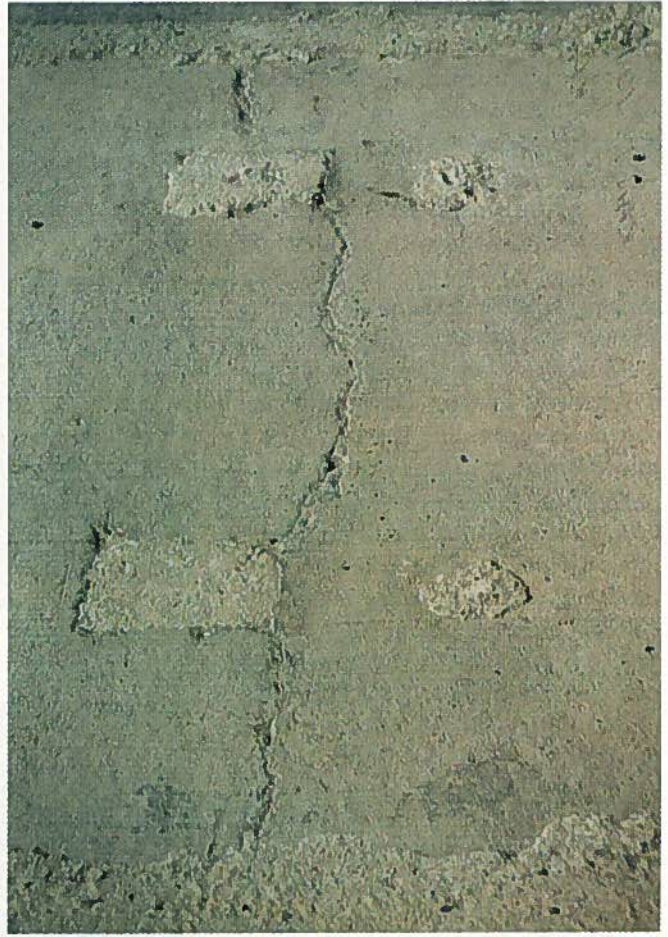
Fig. 37. Cracks between shear pockets, Dalton Highway Bridges, Alaska.
