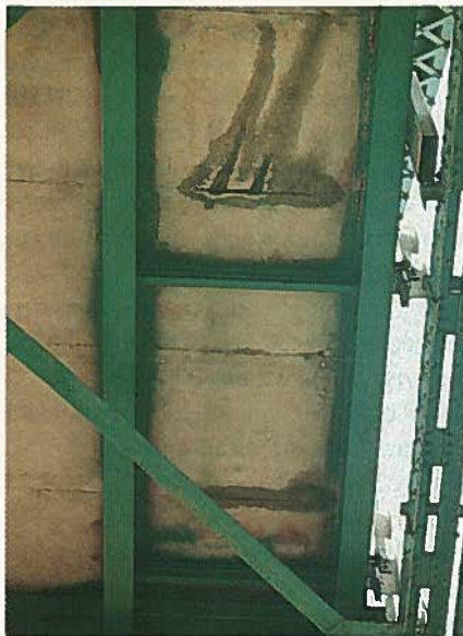
Fig. 2. Condition of bridge deck viewed from below, Seneca Bridge, LaSalle County, Illinois.
