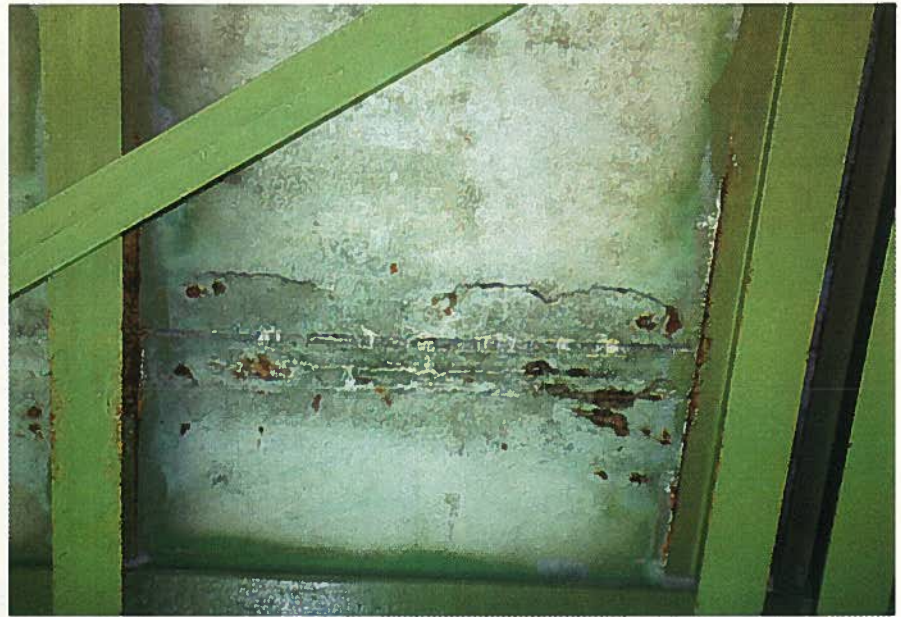
Fig. 30. Spalling underneath bridge deck, Cochection Bridge, Sullivan County, New York.
