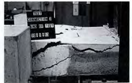
Fig. 21. The end of Test A on connection Type 3 (view of side of end of unit).
