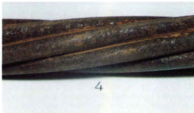
Photo 4. Strand surface before cleaning.
