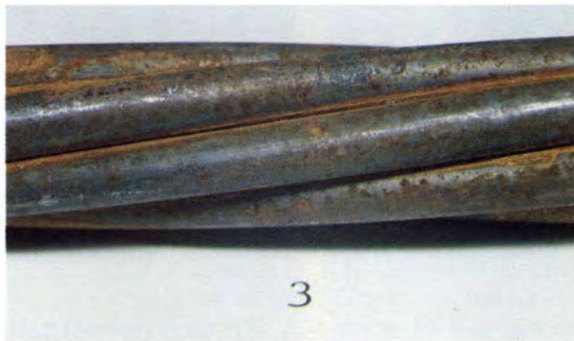
Photo 3. Strand surface before cleaning.
