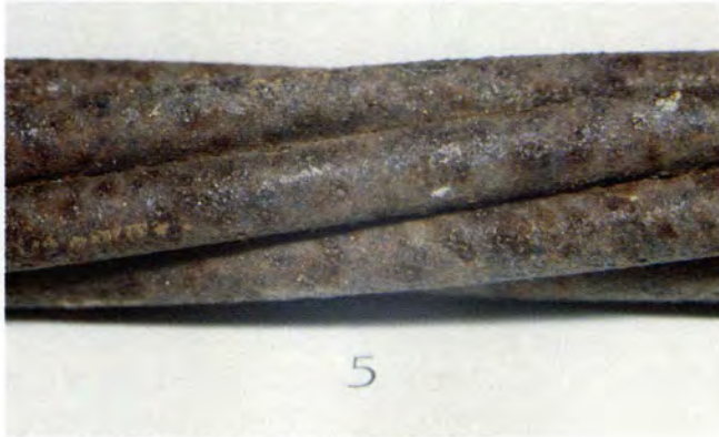
Photo 5. Strand surface before cleaning.
