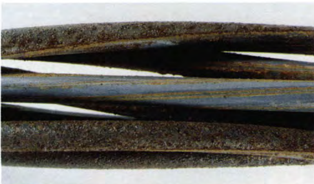
Photo 8. Strand surface before cleaning.
