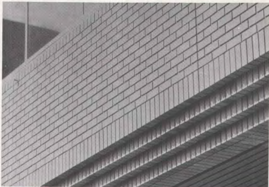
Fig. 21. This second floor spandrel was produced as a single pour operation and shows crisp definition.
