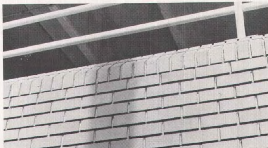
Fig. 20. The concrete laitance is not evident when the total panel is viewed.
