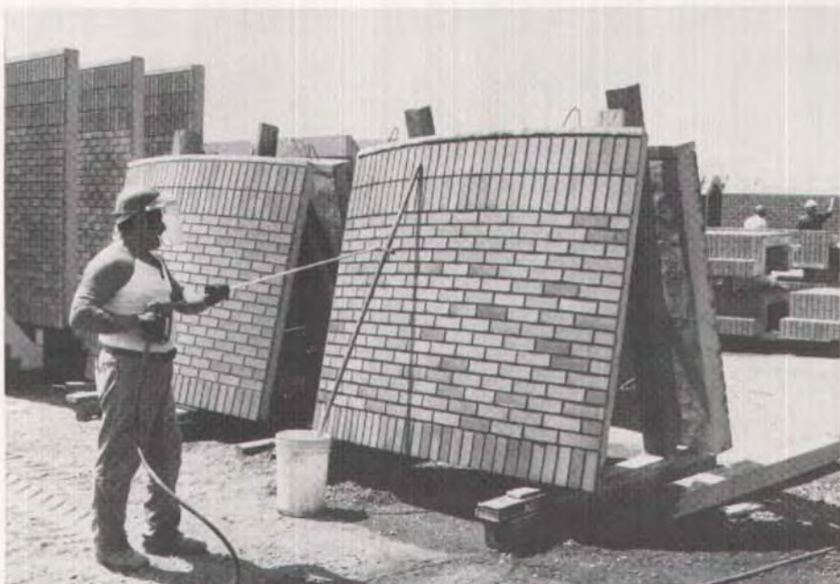
Fig. 16. Spray washing is performed while the rubber formers remain in the joints to avoid removing unset laitance.
