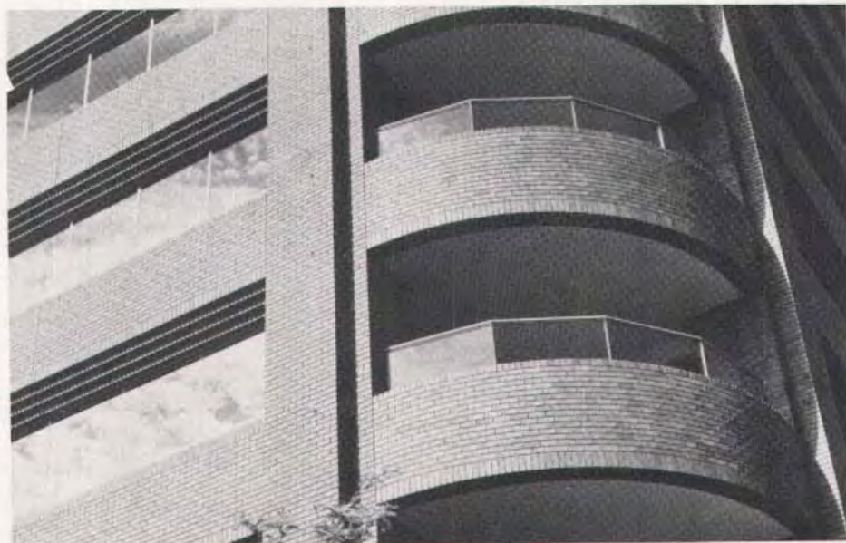
Fig. 6. C-shaped spandrels, U-shaped column covers and curved-on-plan spandrels with brick veneer finish.
