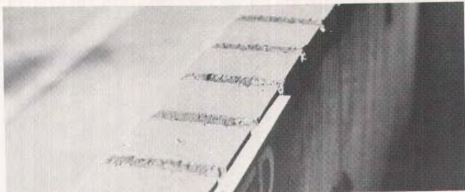
Fig. 18. Concrete laitance is clearly seen upon close inspection of joints.
