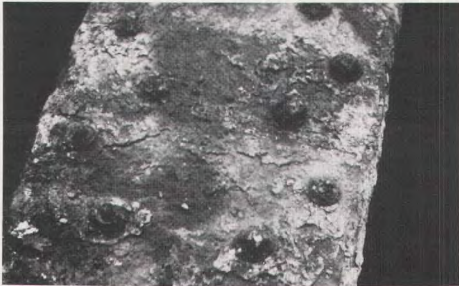
Fig. 55. Deteriorated condition of bridge girder top flange, Santa Fe Railway.
