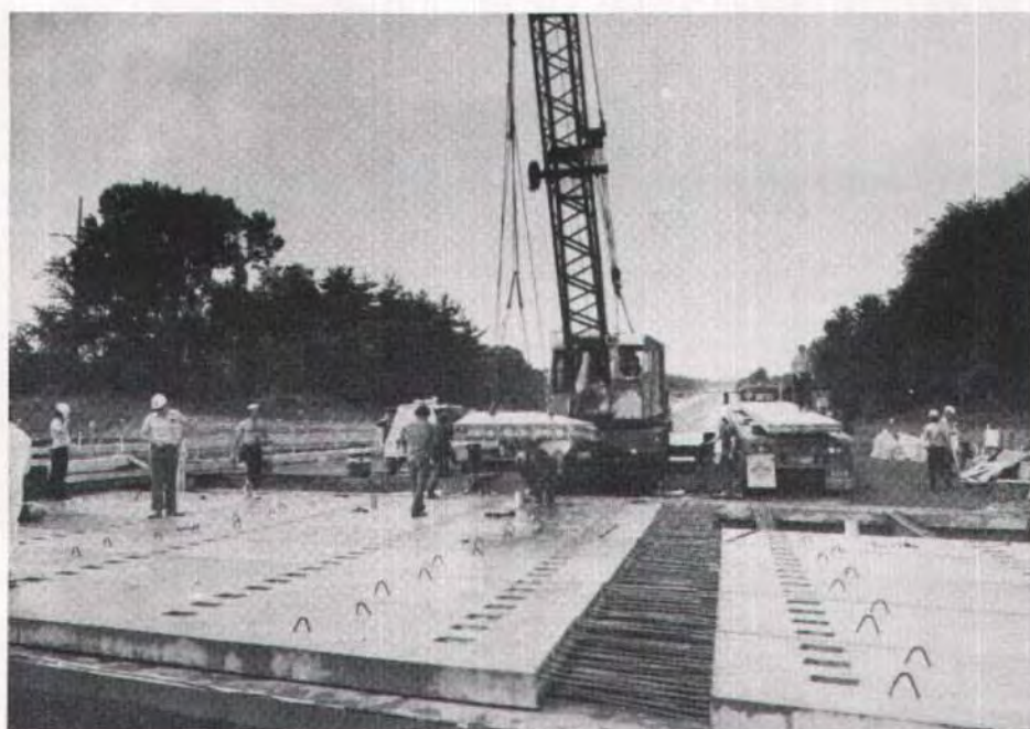
Fig. 21. Placement of 21 ft (6 m) wide panel, and longitudinal joint, Krum Kill Road Bridge.
