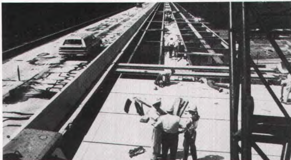
Fig. 24. Placement of new precast panel deck and deteriorated condition of old deck (Clark Summit Bridge).
