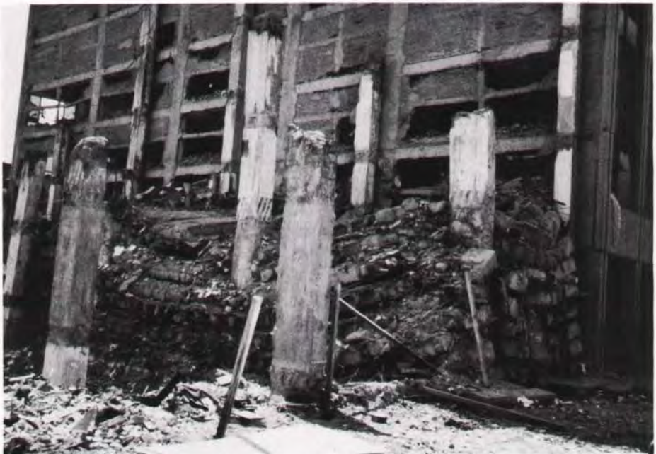
Fig. 4. Columns protruding above pancaked floors failed in punching shear of a flat slab multistory building.
