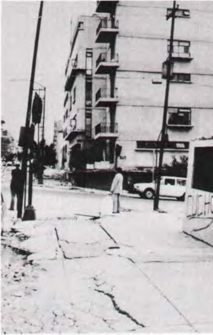
Fig. 7. Building sunk relative to sidewalk.
