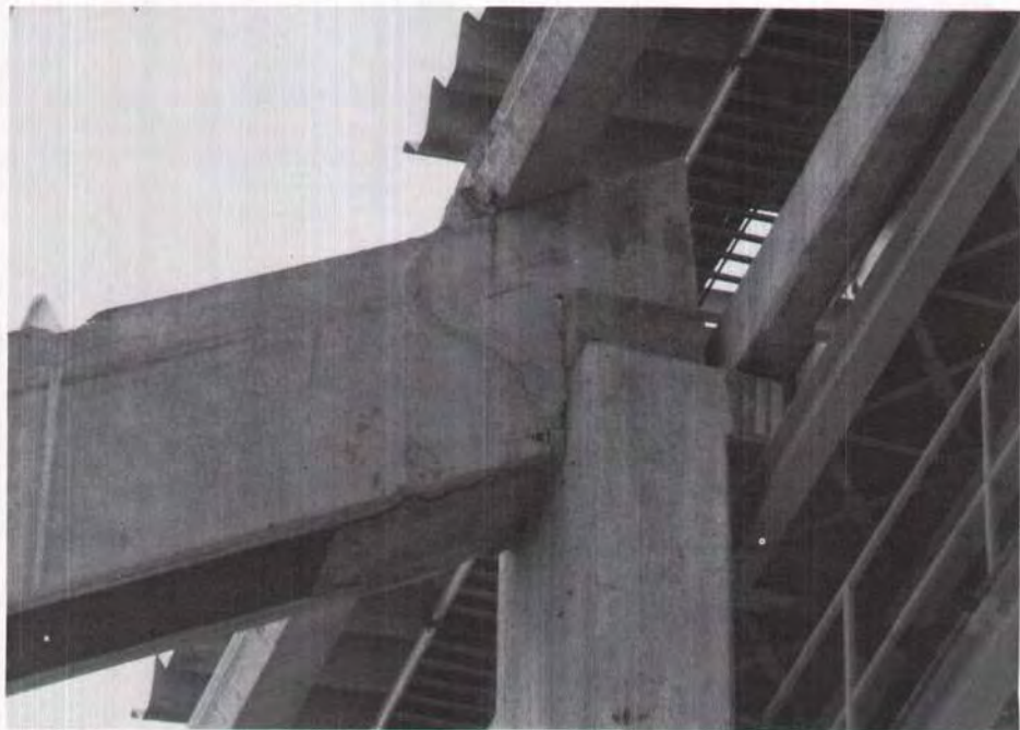
Fig. 20. Shear crack in roof beam.
