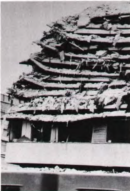
Fig. 3. Pancaked multistory building.
