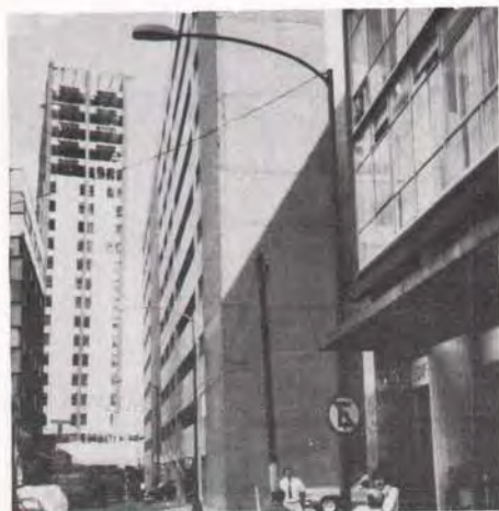
Fig. A8. Ten-story parking garage on Flamingo Avenue. In background is the tilted twenty-one story steel structure.
