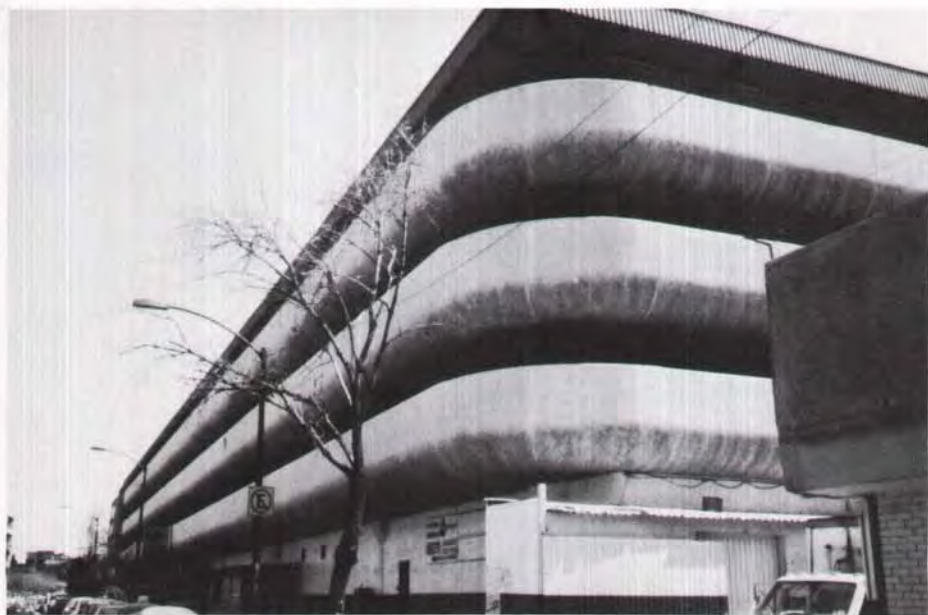
Fig. A5. Four-story parking garage in the zone of maximum damage.
