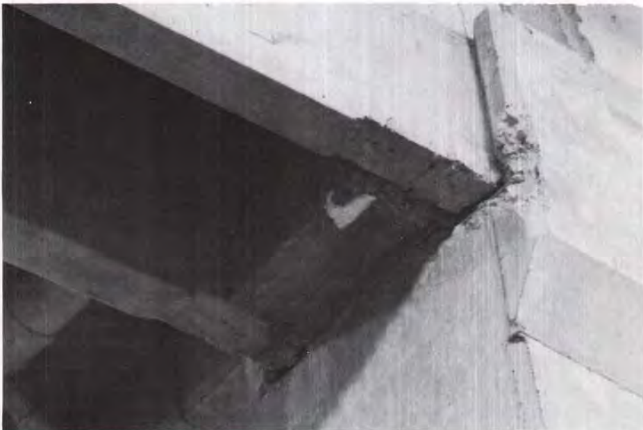
Fig. B4. Beam shifted 20 cm (8 in.) at top of column.
