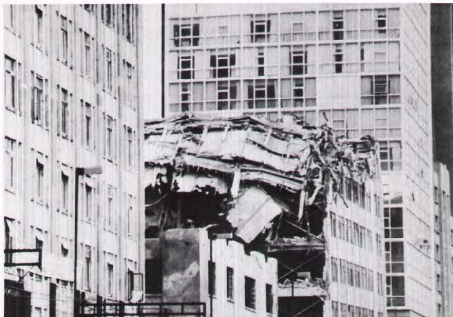
Fig. 5. Collapsed upper stories.
