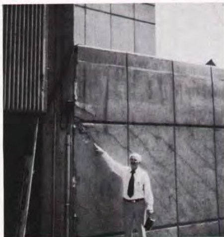
Fig. A4. Cracked buttressing wall at garage entrance.
