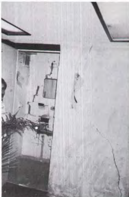
Fig. A2. Cracking of masonry partitions in adjacent building.
