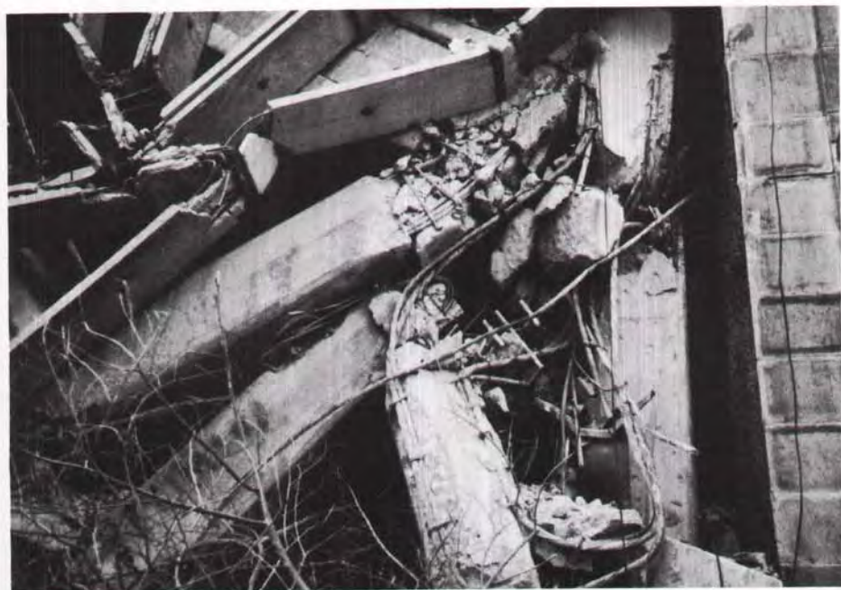
Fig. 15. Detail showing partially collapsed seven-story parking garage at Carranza St.
