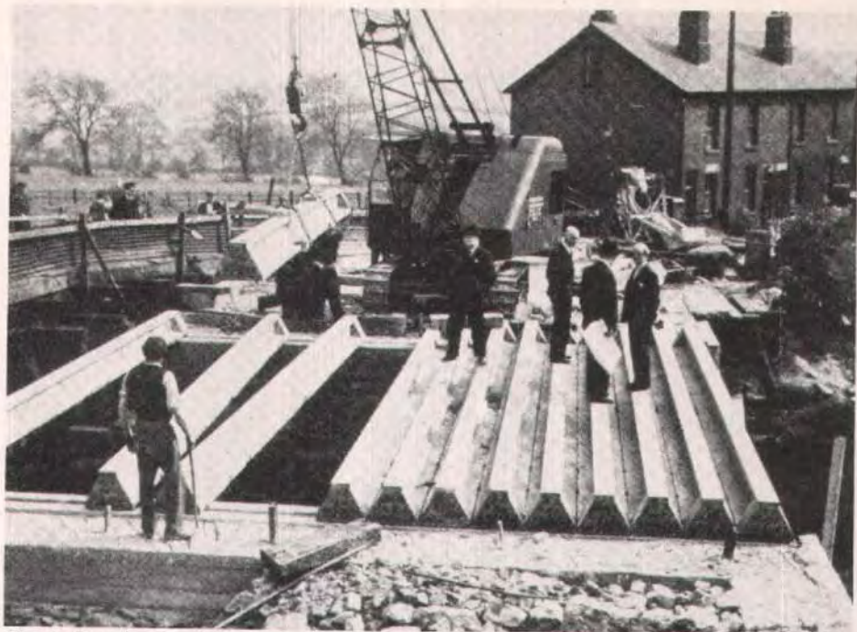
Fig. 4. Erecting partially prestressed inverted T beams for the Gilroyd Bridge on the Manchester-Sheffield railroad line in 1949. Dr. Paul Abeles is on the right.
