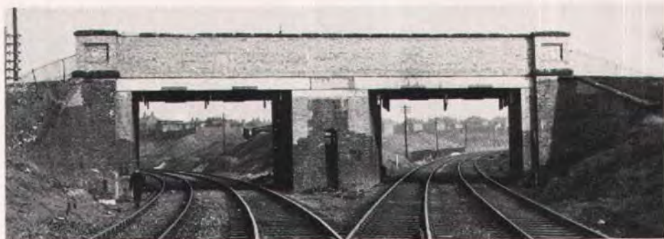
Fig. 3. Masonry arch bridge after reconstruction using composite partially prestressed concrete deck for overhead electrification. Two-span structure at 31 ft (9.5 m) was built for British Railways in 1951 (Gorton-Manchester line).
