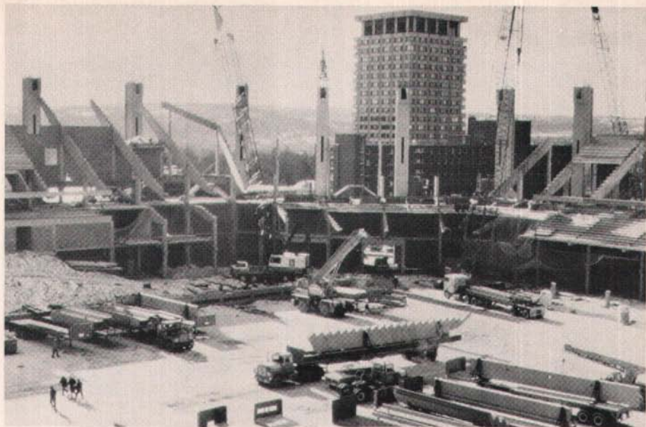
Construction of the stadium bowl. The interior arena space lends itself readily for storing the precast columns and bents.
