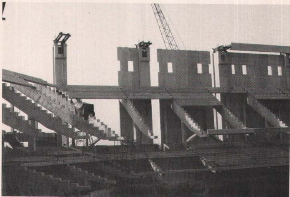
Erection of the exterior wall system. Openings in the wall panels are for air intake dampers. Note the cantilevered steel dunnage to receive the inside precast flange for the "U" shaped ring beam.
