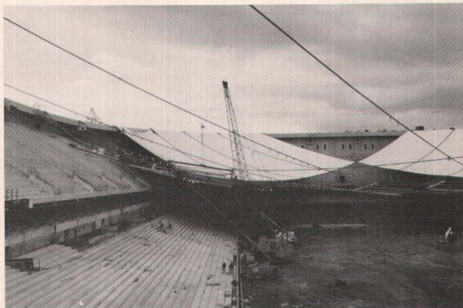
Erection of the roof fabric over the strung roof cables. The gig supported by an overhead cable spools out the fabric roof panels which are clamped to the roof cables.
