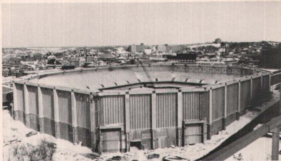
The erected stadium bowl 8 months after ground was broken. The precast double tees and columns create a clean and maintenance free exterior.
