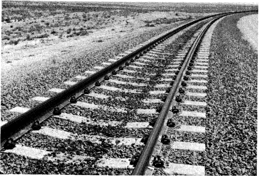
Fig. 27. Concrete tie track on the Facility for Accelerated Service Testing.
