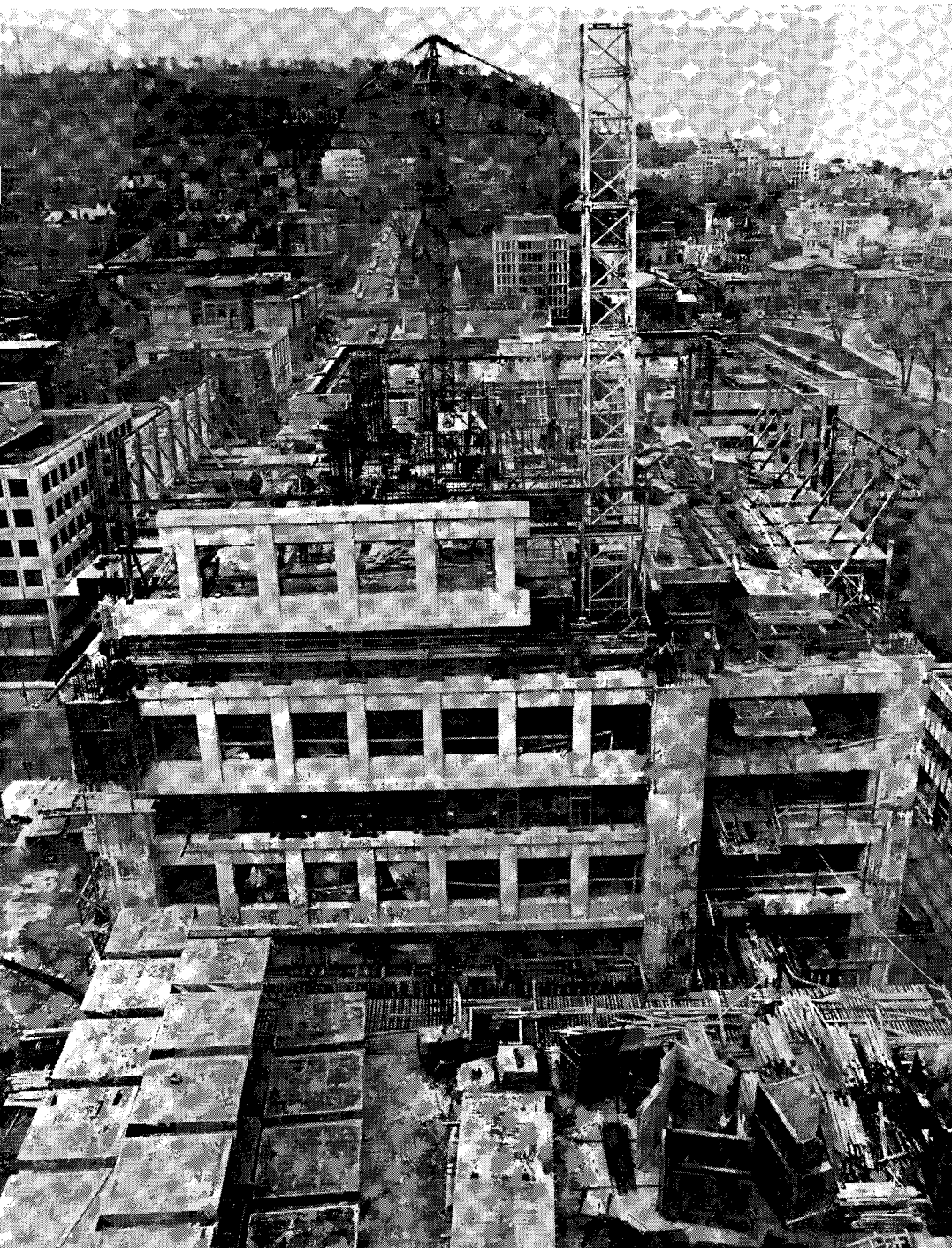
Fig. 15. Overall shot of construction operations from south side. The truss on the west wall is in place, diagonal bracing is prepared on the east wall, and the south wall truss is partially erected.
