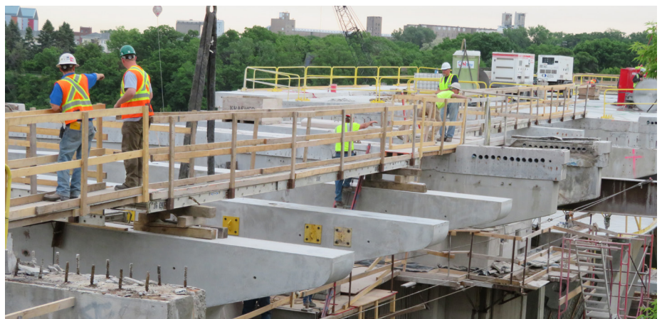
Project Name: Franklin Avenue Bridge • Owner: Hennepin County • Contractor: Kraemer North America • Engineer: Hennepin County and HNTB Engineers
