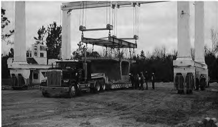
Fig. 11. A lowboy truck carries segments from the casting yard to the project site 35 miles (56 km) away.
