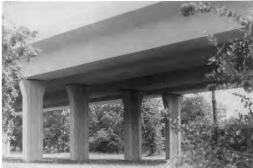
Fig. 18. A view from underneath the completed structure where four precast box girder superstructure sections are connected. The smooth, closed shape of the superstructure and the pleasing pier shapes insure compatibility with the parks, bike paths, playgrounds and tennis courts that the city is constructing under and around the bridge.
