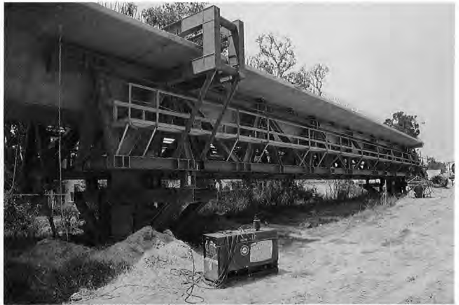
Fig. 13. Most of the bridge was erected by the span-by-span method of construction utilizing erection trusses supported by falsework at the piers.
