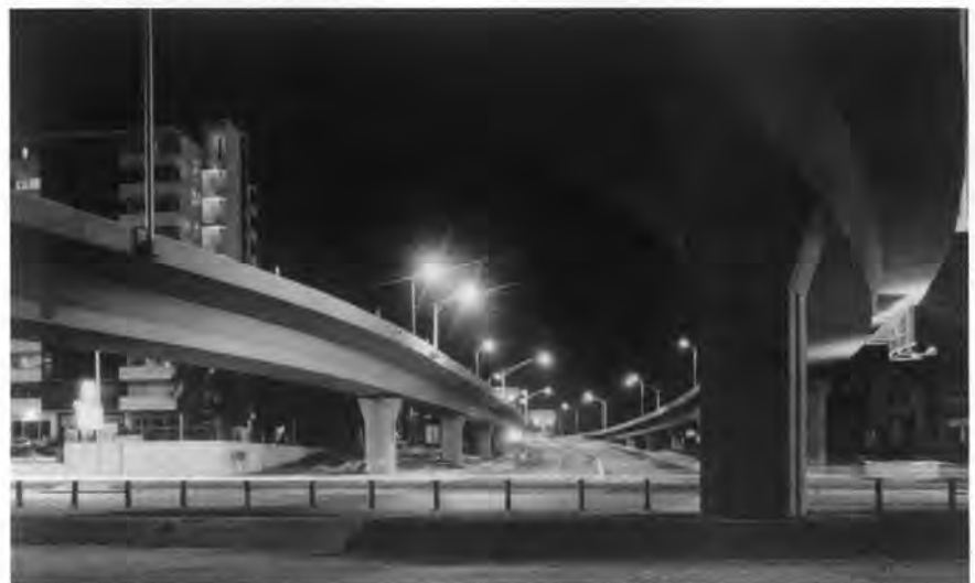
Fig. 20. The completed structures at night. These precast concrete structures represent over 616,600 sq ft (57344 m 2 ) of elevated interstate. The total project cost was $40.2 million. This precast concrete design saved $4.2 million over a cast-in-place concrete alternate.
