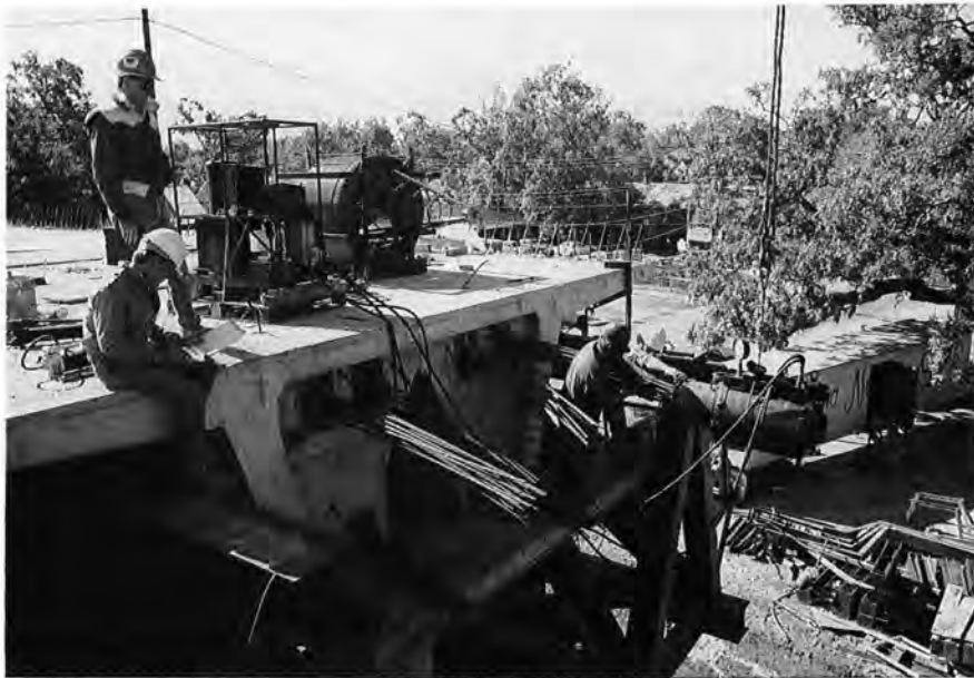
Fig. 15. Post-tensioning of the main longitudinal tendons completes the span erection cycle and allows the erection trusses to be moved to the next span.
