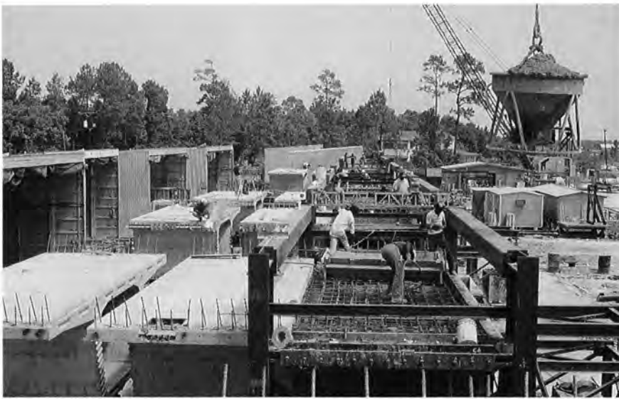
Fig. 10. Typical segment being cast. Steel frame surrounding the casting machine anchors the transverse pretensioning. The segment just to the left of the casting cell is in the match cast position, while the segment on the far left is awaiting transportation to the storage area.
