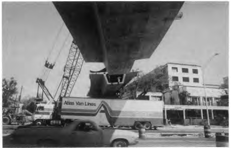
Fig. 17. Traffic continues to move during precast concrete segmental cantilever construction of the 180 ft (54.9 m) spans across U.S. 90.
