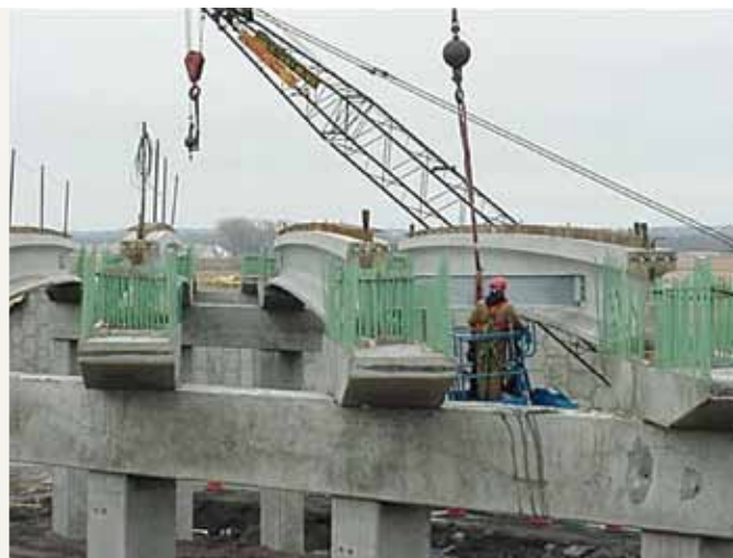
Figure 10. The camber is visible in the Nebraska Clarks Bridge because of the extended time between prestress release and erection.
