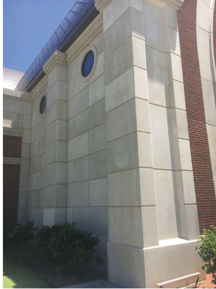
Design-assist was used in St. George Catholic Church to create an aged limestone-and-brick motif. Courtesy of www.toddlandryphotography.com .
