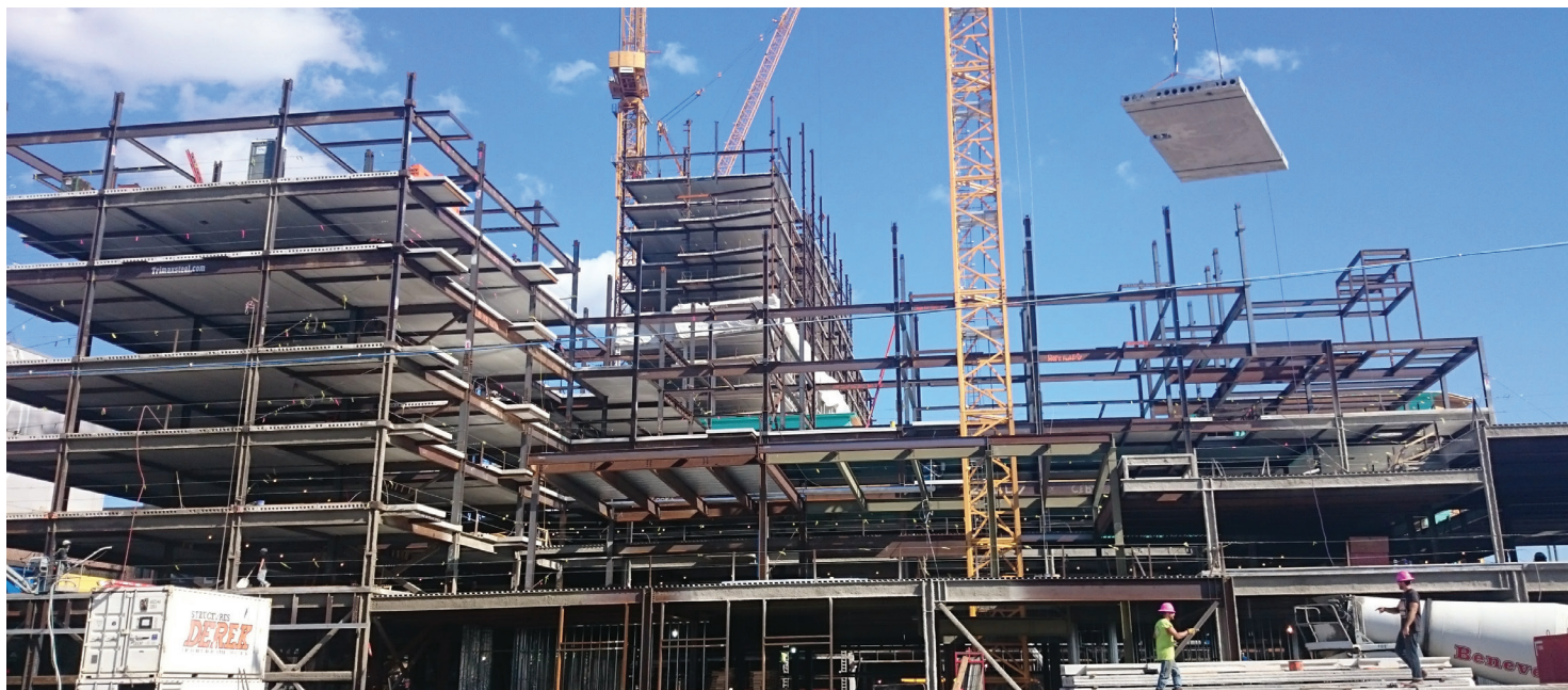
Hollow-core structural flooring is being erected for the Assembly Row mixed-use complex in Somerville, Mass. J. P. Carrara & Sons Inc. provided the hollow-core, which made it possible to erect the structural slabs in winter and provided lower floor-to-floor heights than would have been possible with conventional structural steel. Courtesy of J. P. Carrara & Sons Inc.
