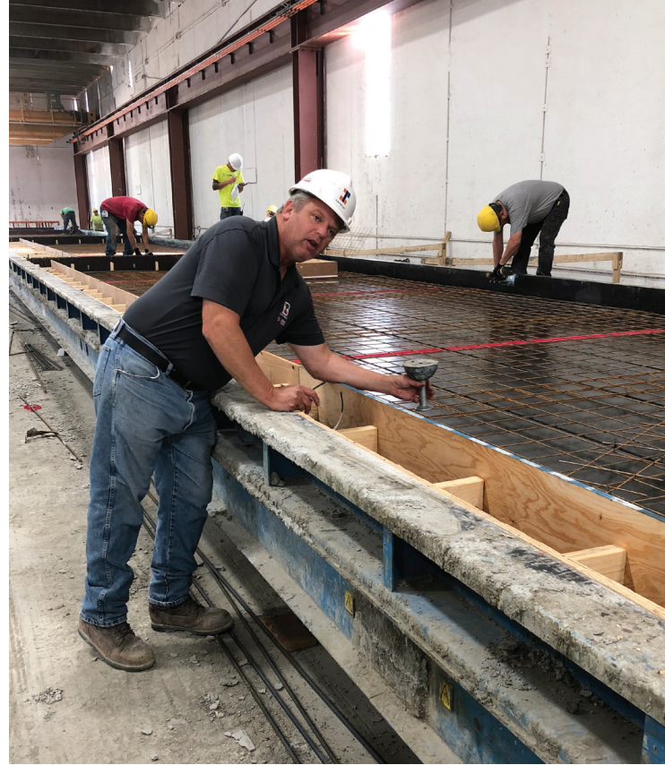
Don Caithamer, QA manager at Illini Precast, shows PCI employees where hardware will be cast in the panel during a tour of Illini's plant in Romeoville, Ill. Courtesy of Nikole Clow.
