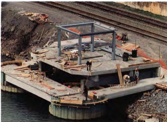
Stair and ramp sections used on the central pier consist of single precast units 32 ft (9.7 m) in length cast in formwork up to 7½ ft (2.3 m) tall.
