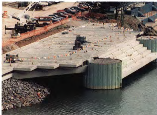
The boat landing comprises precast concrete double tees, flat slabs, bleacher seats, rectangular beams, raker beams, and inverted tee beams.
