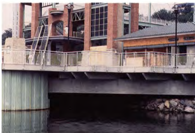
Double tees, cantilevering by as much as 15 ft (4.6 m), form the walkway of the central landing area.
