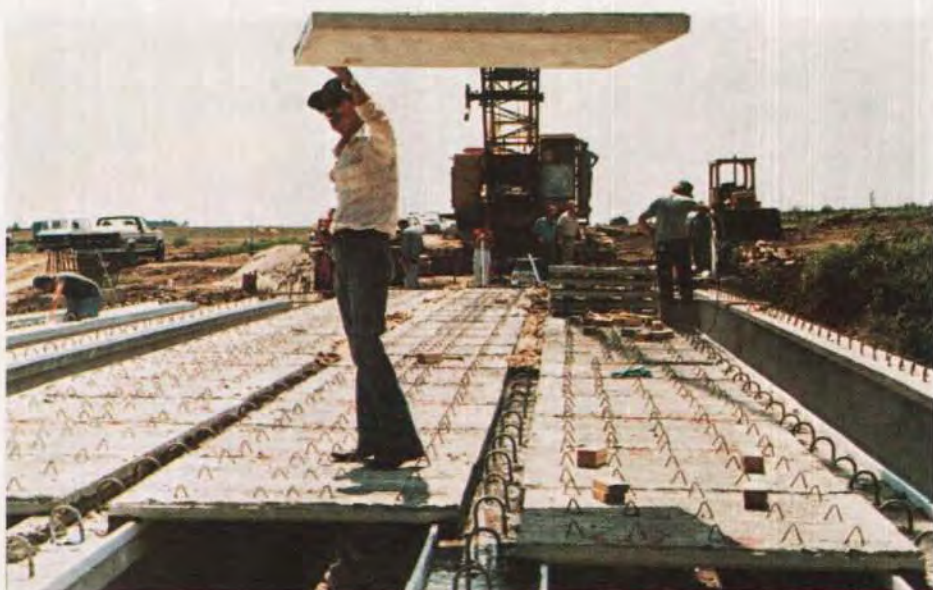
Fig. B12. Placing 2½ in. thick panels on a 42 in. precast prestressed concrete I beam bridge in central Illinois. The EPS form was cut to the required fillet height. It is generally advisable to place grout while placing panels to avoid air pockets.
