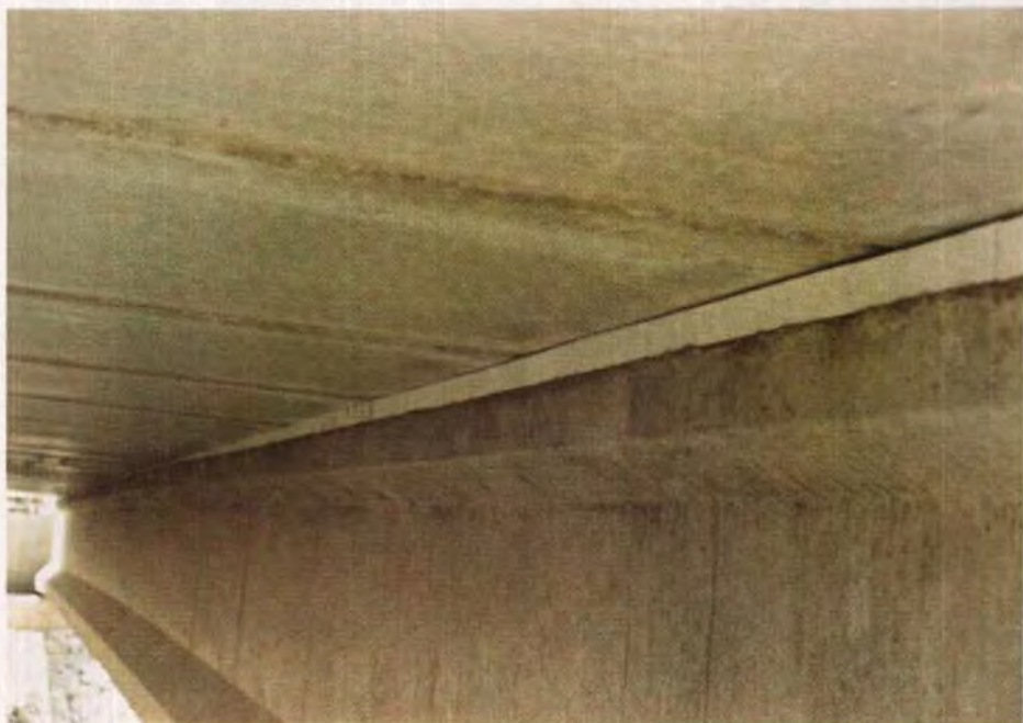
Fig. B13. The panels and the EPS are in place on the structure shown in Fig. B12.
