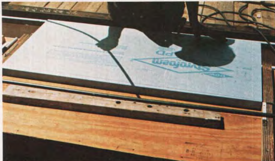
Fig. B2. The EPS being hot-wire cut to the correct fillet height before it is attached to the top flange.
