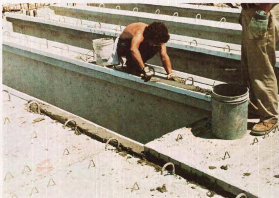
Fig. B14. The workman is placing grout ahead of the panel setting.
