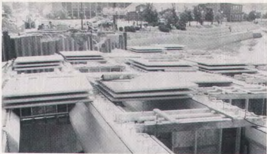
Fig. 3. This view of the Colfax Bridge over the Saint Joseph River in South Bend, Indiana shows the diaphragms cast in place. The panels are stored on the beams to speed the final placement. These panels were placed on a fibrous material. An effective detail, shown below, is being used in a number of states, with good results.
