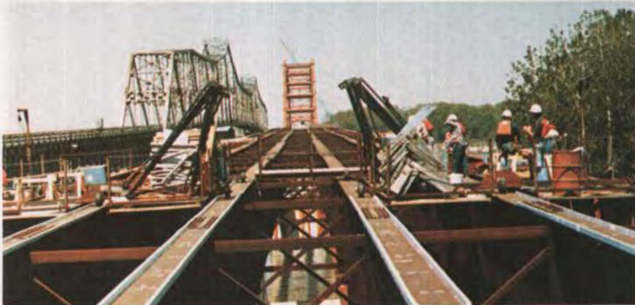
Fig. B1. Looking west, the high density expanded polystyrene foam (EPS) on 10 ft deep steel plate girders can be seen. Removing wood forms, over the water in this situation, would have been difficult.
