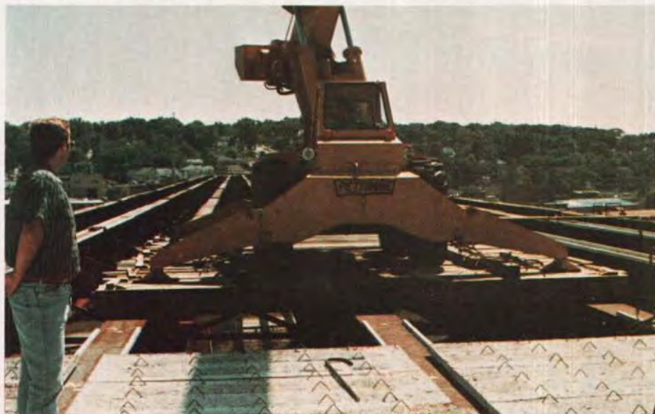
Fig. B11. An 18 span 66 ft wide steel plate girder high level structure at Lemont, Illinois crosses a highway, a ship canal and a railroad. This structure required 190,000 sq ft of 2½ in. thick x 48 in. wide panels. Because of curve at each end, the panels were bevelled on each side. The small crane set the panels after a large crane unloaded the trucks below.
