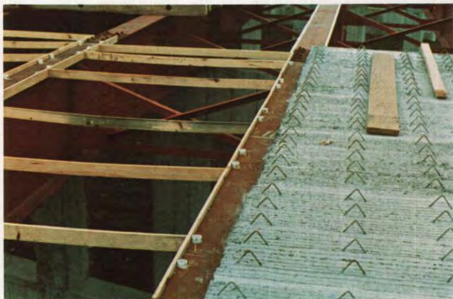
Fig. B6. On this eleven span steel plate girder bridge over a railroad in St. Clair County, Illinois, the narrow flange did not allow the use of EPS. PVC pipes were cut to fillet height and glued to the flange. 2 x 4 in. and 2 x 6 in. boards were wedged (not nailed) against the side of the flange to hold the grout bed in place after panels were set. Stripping was simple. Hooks with long handles were used from the ground to pull out the bowed transverse wood wedges.
