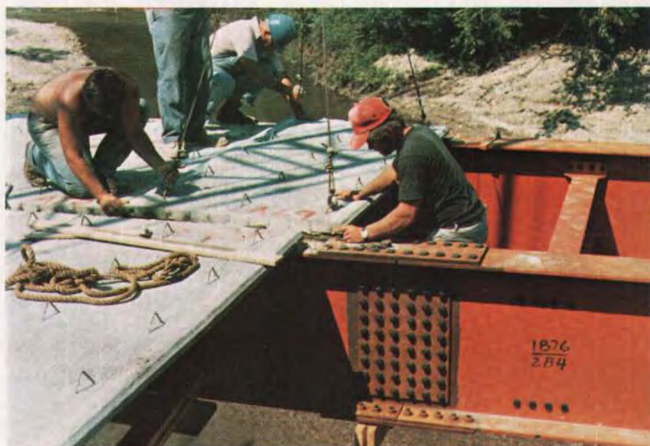
Fig. B10. Placing panels at steel beam splice where fillets are small. Notice that small bolt head must be on top of flange plates. Common ironworker practice is to put bolt head on underside of top flange.
