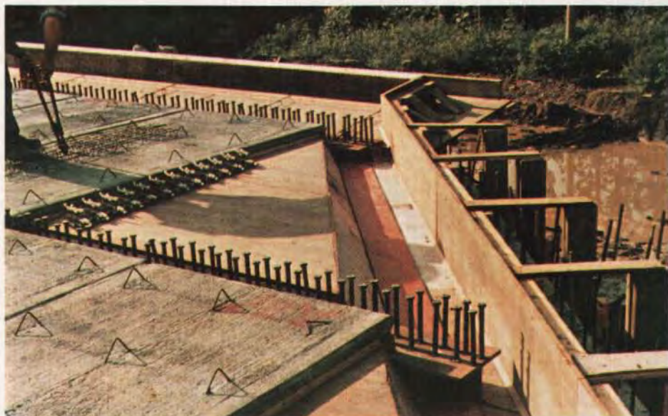
Fig. B9. Details at skewed end of a 33 WF steel beam three span bridge in Bureau County, Illinois. The 45 degree skewed end section was formed and poured full depth in the field.
