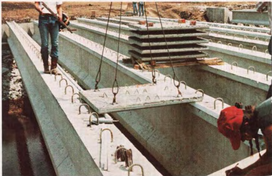
Fig. B15. Placing panels on a precast prestressed concrete I beam structure. Note how a group of panels are unloaded from trucks and stored on the beams before lifting each one into place.
