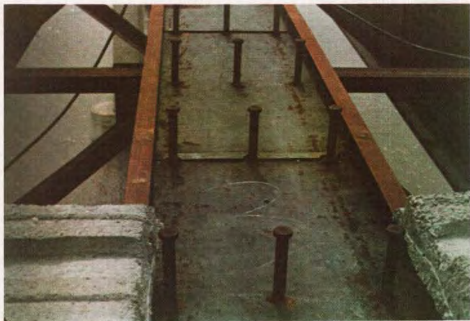
Fig. B16. 3½ in. thick panels on a steel plate girder bridge near New Orleans, Louisiana. These are set on steel angles prefabricated to proper fillet height shown in Fig. B2.
