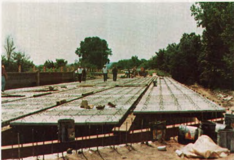
Fig. B8. An overall view of the same structure shown in Fig. B7 (above). The panels are in place ready for steel shear connectors, reinforcing steel and deck concrete.
