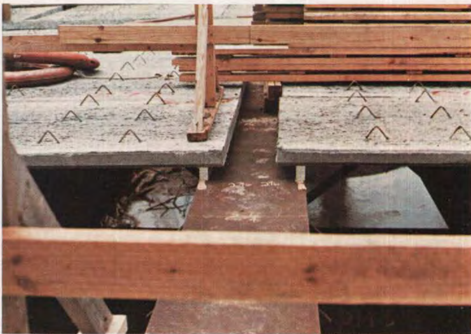
Fig. B3. The panels supported on the EPS, before placing the deck concrete.
