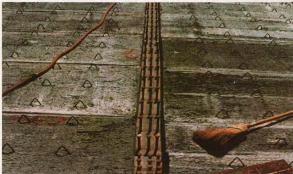
Fig. B5. The deck panels and steel shear connectors in place ready for reinforcing steel and deck concrete.
