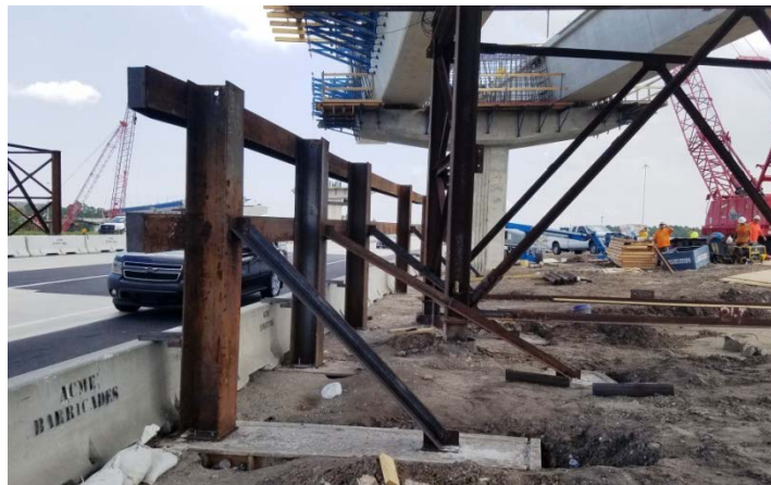
Fig. 7: Crash Rail Protection Adjacent to I-95 Traffic
