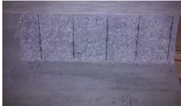
137 138 Fig. 4 Beam web after cover removal 139
