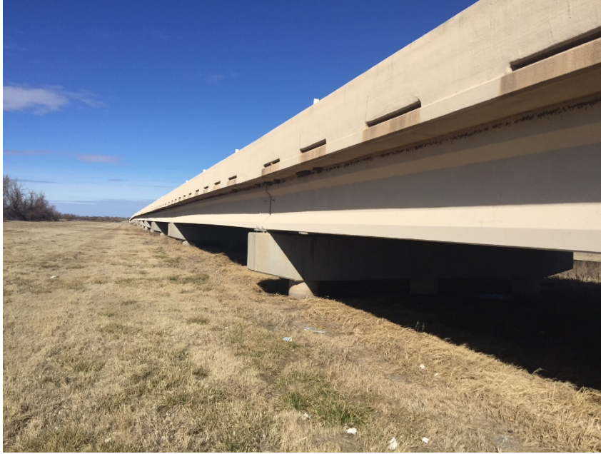
Figure 1. North Canadian River Overflow Structure, John Kilpatrick Turnpike, Oklahoma, consistently of nineteen 103'-4" spans in both northbound and southbound directions with Type IV Girders spaced at 8'-0" centers.
