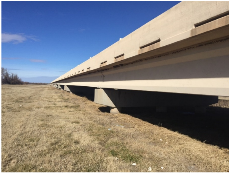
Figure 1. North Canadian River Overflow Structure, John Kilpatrick Turnpike, Oklahoma, consistently of nineteen 103'-4" spans in both northbound and southbound directions with Type IV Girders spaced at 8'-0 centers.
