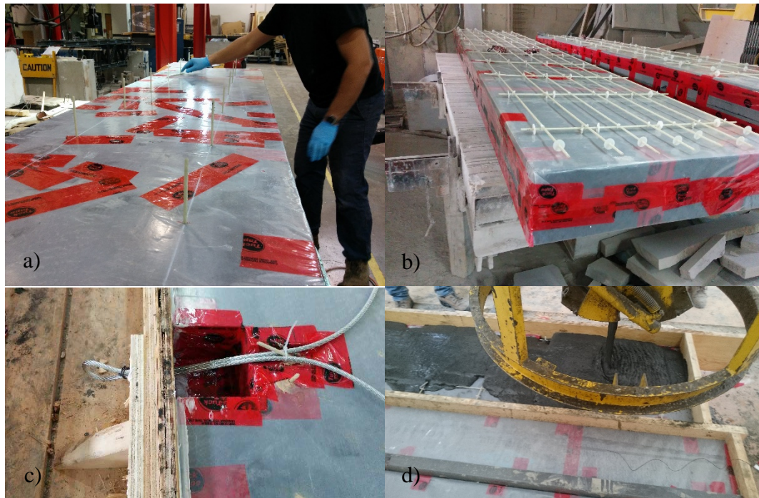
Fig. 3 Fabrication of concrete double wythe insulated panels: a) inserting GFRP connectors into the foam; b) assembling the GFRP grid; c) voids for the lifting cables; d) casting concrete
