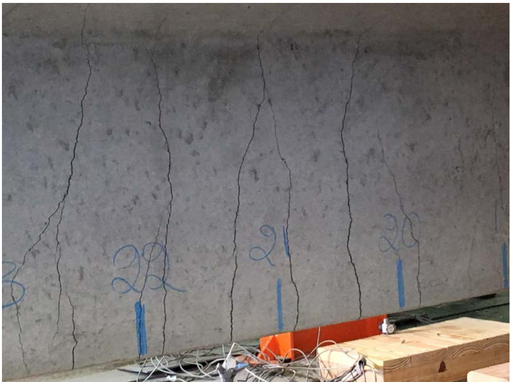
256 257 Fig. 18. Widening of the cracks and formation of new cracks during ultimate flexural test
