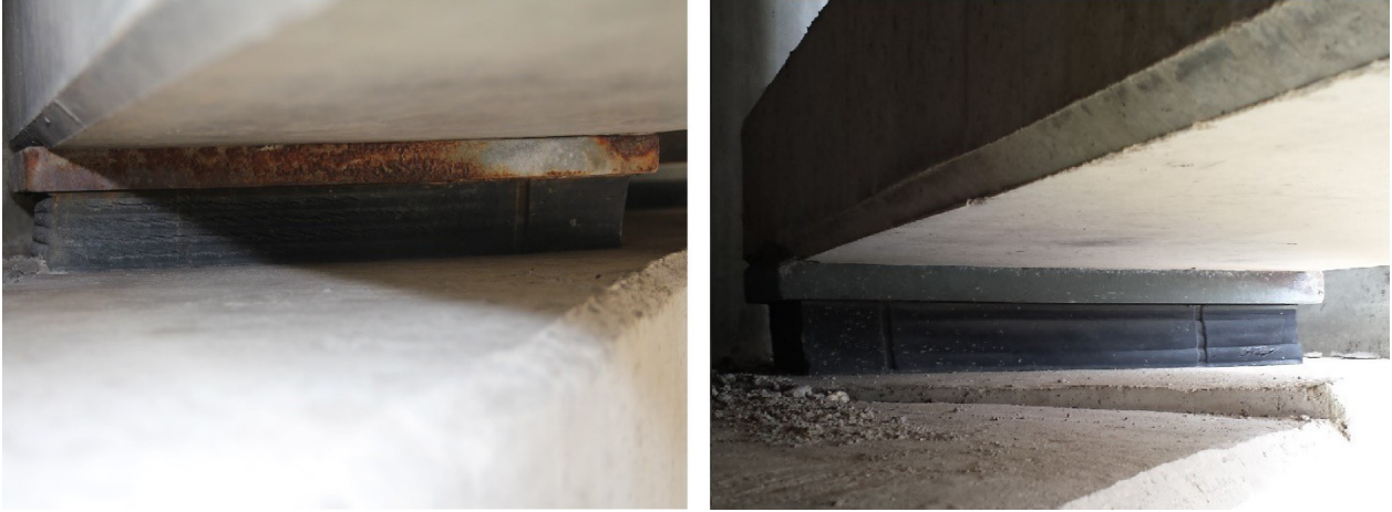
(a) (b) Fig. 10 (a) Lateral displacement, and (b) rotation of the bearing for 52° skew.
