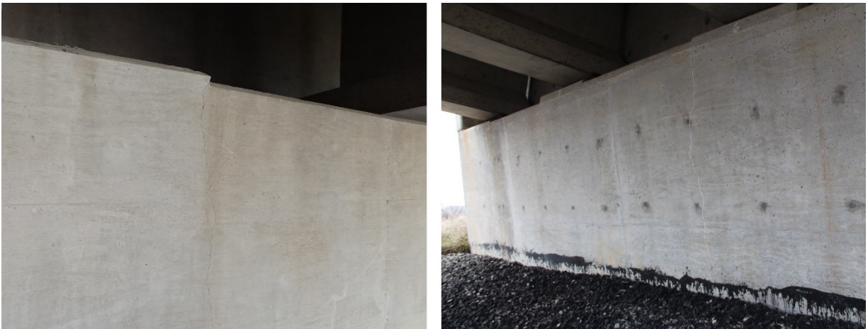
(a) (b) Fig. 11 Vertical abutment cracks for bridges with (a) 52° skew, and (b) 0° skew.
