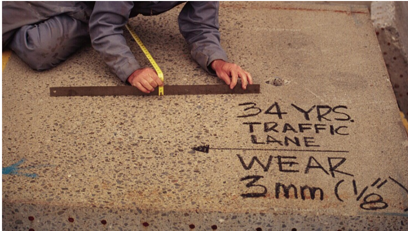
Fig. 2 Photograph of deck section removed from the Boulevard Bridge in 1993.
