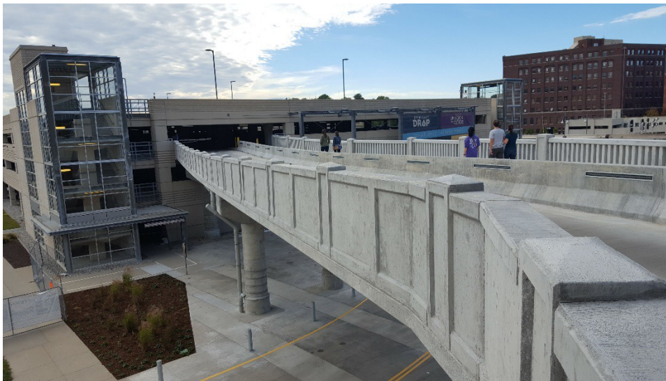
Figure 6 – “Warped” Bridge Deck Drainage
