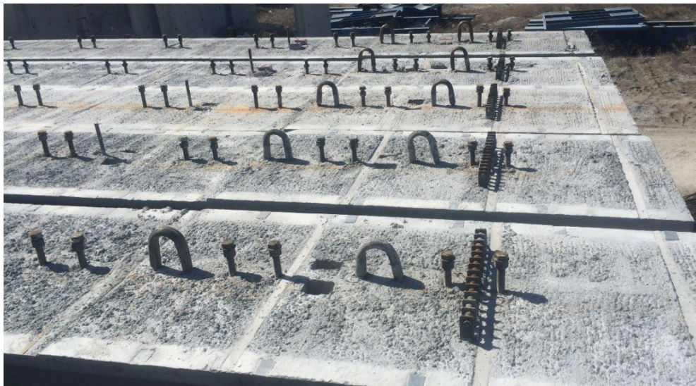
Figure 3: Precast/prestressed concrete NU1800 girders for the new precast concrete deck system Deck Production
