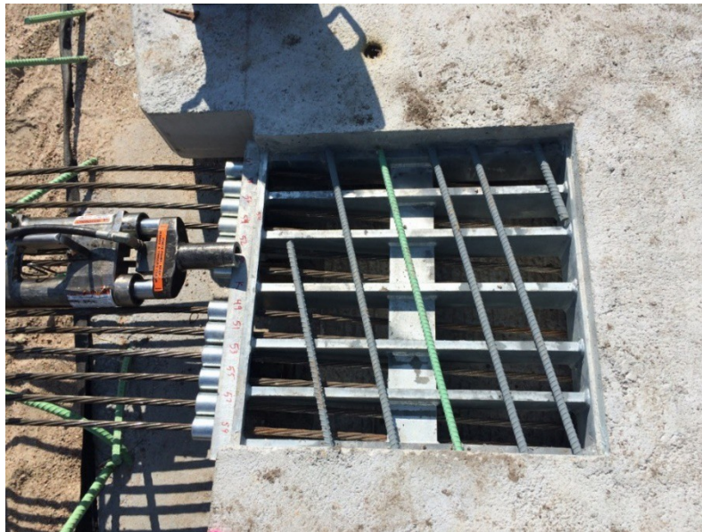
Figure 12: Post-tensioning strands and anchor block.
