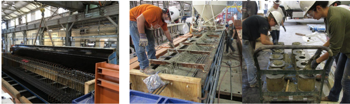
(d) Installing the side forms (e) Casting the beam and match-curing specimens
