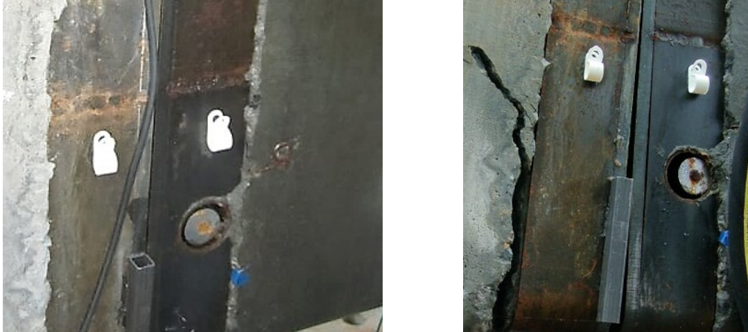
216 217 Fig. 12 – Test 1 location of locking pin prior to (left) and after (right) load tests 218 219
