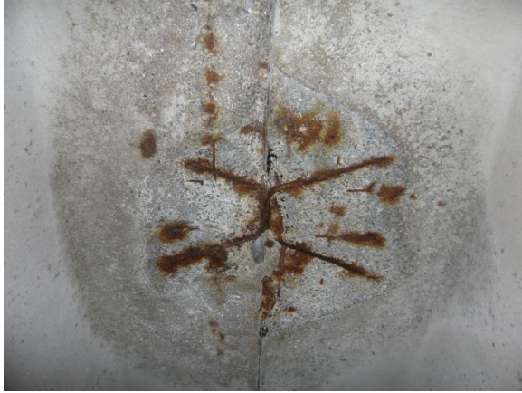
Figure 3. Concrete spall below flange-to-flange connection that is corroding in field-topped deck
