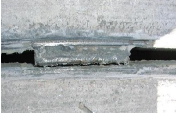
Figure 8. Fractured weld at flange-to-flange connection
