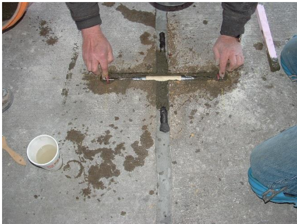
Figure 14. Stainless steel bar with sleeve installed in slotted opening, named “dog-bone” repair
