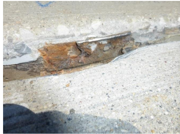
Figure 9. Fractured faceplate at flange-to-flange connection
