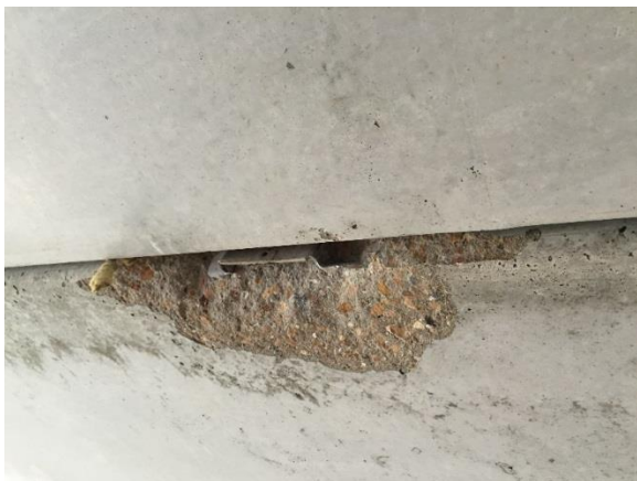
Figure 5. Concrete spall below stainless steel flange-to-flange connection in pre-topped deck
