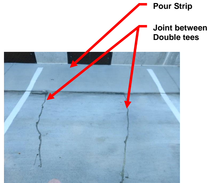
Figure 28. Cracks at end of double tee in line with at stem connections to wall (cracks in pour strips are not visible)
