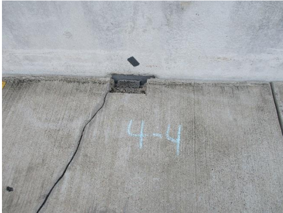
Figure 27. Crack at end of double tee that starts at stem connection to wall
