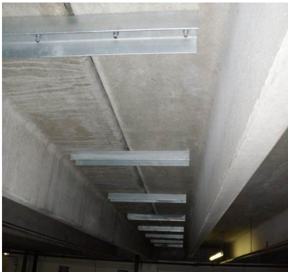
Figure 12. Supplemental steel channels attached to the underside of double-tee flanges
