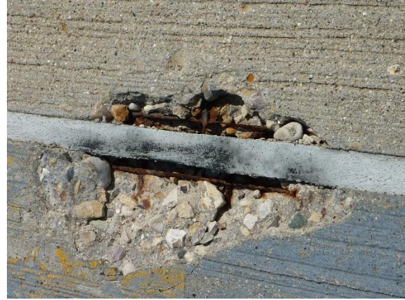
Figure 4. Cracked and spalled concrete above flange-to-flange connection in pre-topped deck
