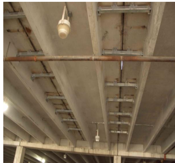
Figure 13. Supplemental steel tubes attached to the underside of double-tee flanges and stems
