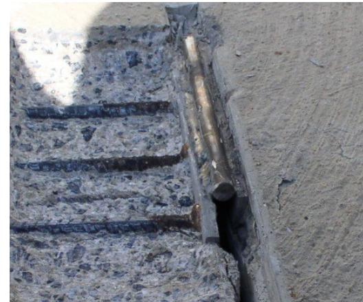
Figure 36 Cracking at concrete and corrosion of rebar due to large weld at stainless steel embedment.
