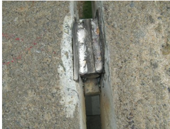
Figure 35 Spall due to welding at stainless steel embedment.
