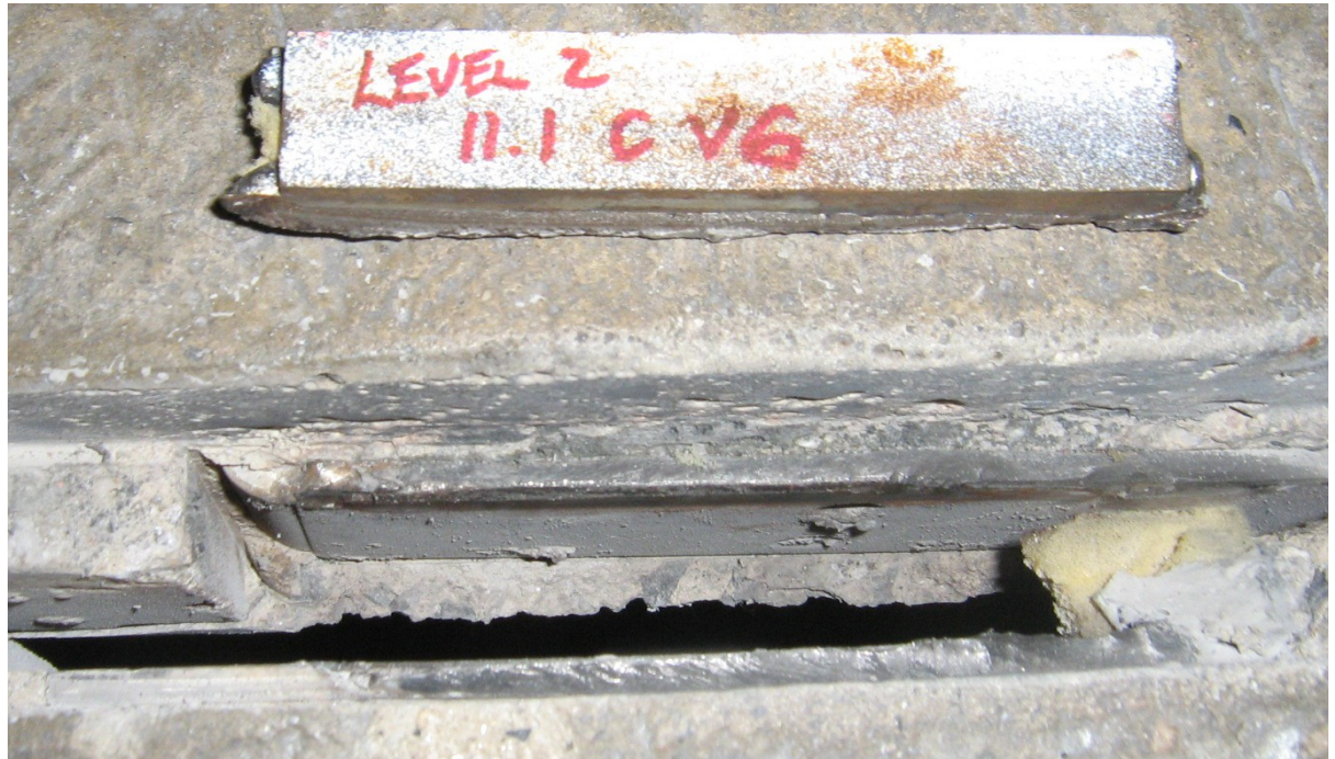
Figure 9 Fatigue fracture at flat erection bar (shown upside-down). Note uniform and burnished crack propagation zone and linear striations at face of weld fracture (red arrow) and abrupt fracture at face of weld (black arrow).
