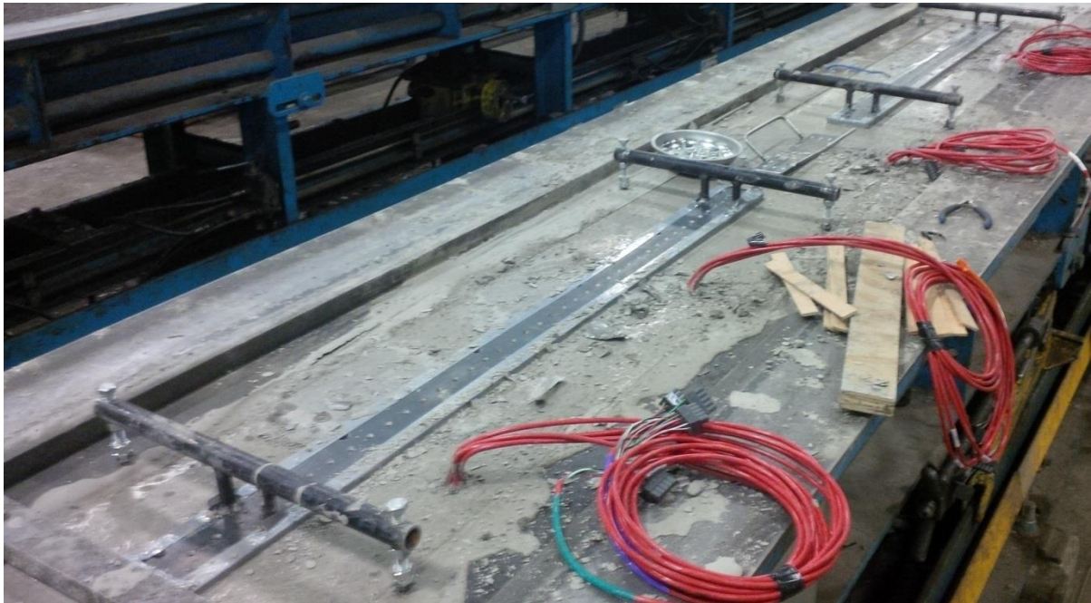
Figure 6: Special steel bars held the brass inserts at one-inch spacing on the concrete surface
