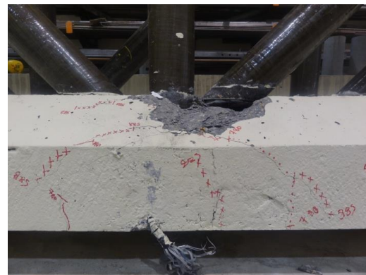
(b) Crushing of Bottom Chord
