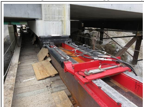
Figure 20: Hydraulic Jacks and Gripper Assembly
