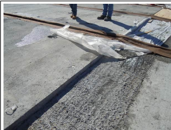
Figure 4: Step due to NEXT Beam Camber
