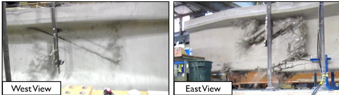
Tx62-3 (South): immediately after shear failure
