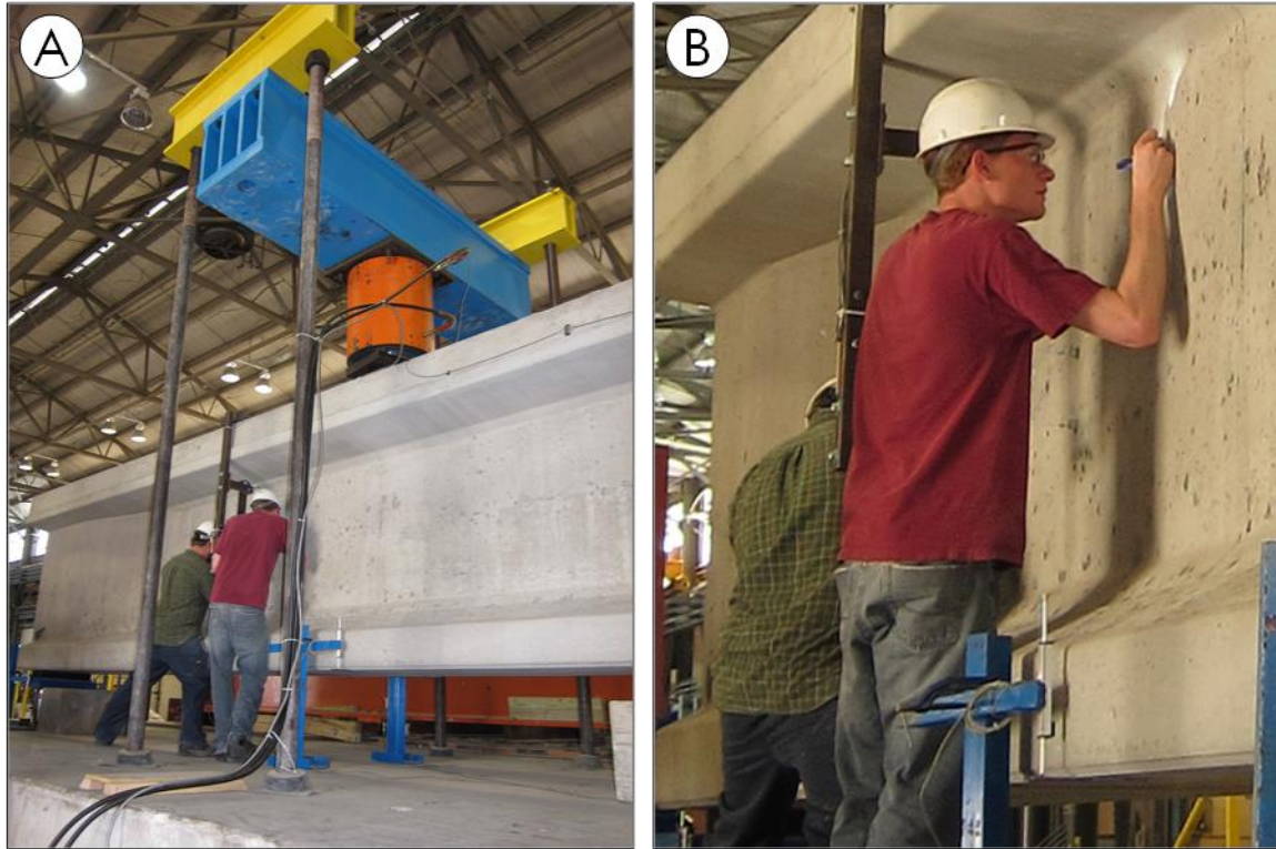
Figure 9: (A) 2,000 kip Load Frame & (B) Crack Mapping between Load Steps
