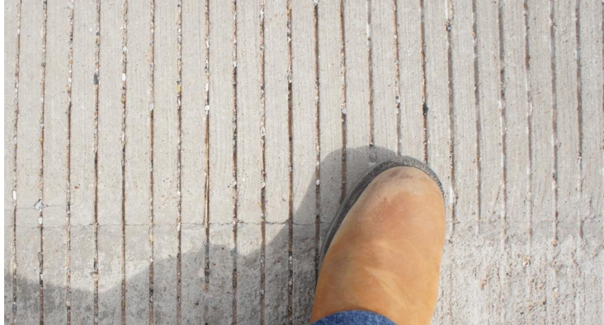
Figure 9. Cold Joint Crack
